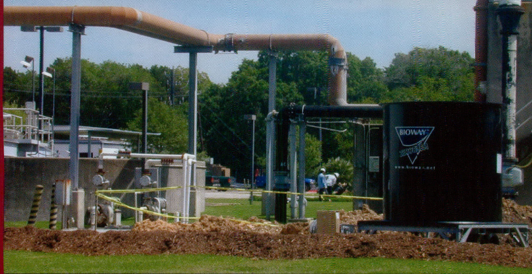
An odor-control system will protect employees and equipment at the headworks
