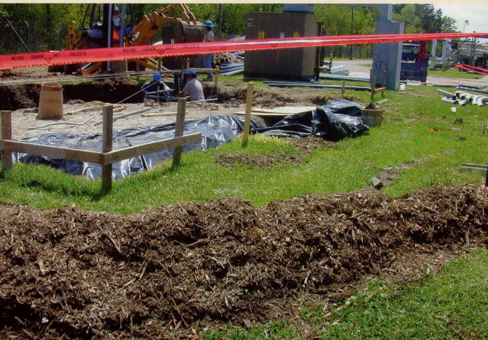
Above: Foundation work is underway at Blackhawk Facility for a new building to house upgraded electrical switchgear. Foreground is a mulch berm being used to control silt runoff during construction. Top right: Mulch-filled plastic rings protect drains in the plant.
