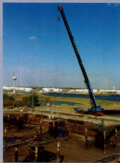
A 120 ton crane was brought in to move components during the basin workover.
