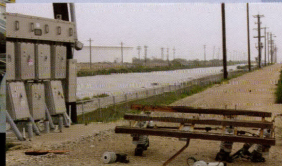
Electric fuses at 40 Acre.
