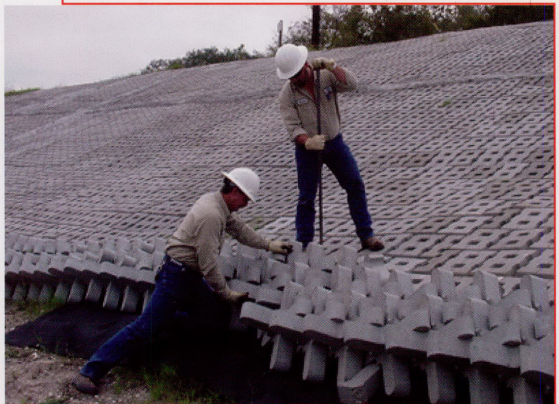
GBRA Coletto Creeek employees install concrete revetment mats as part of an erosion repair project on the Main Dam spillway discharge channel.
