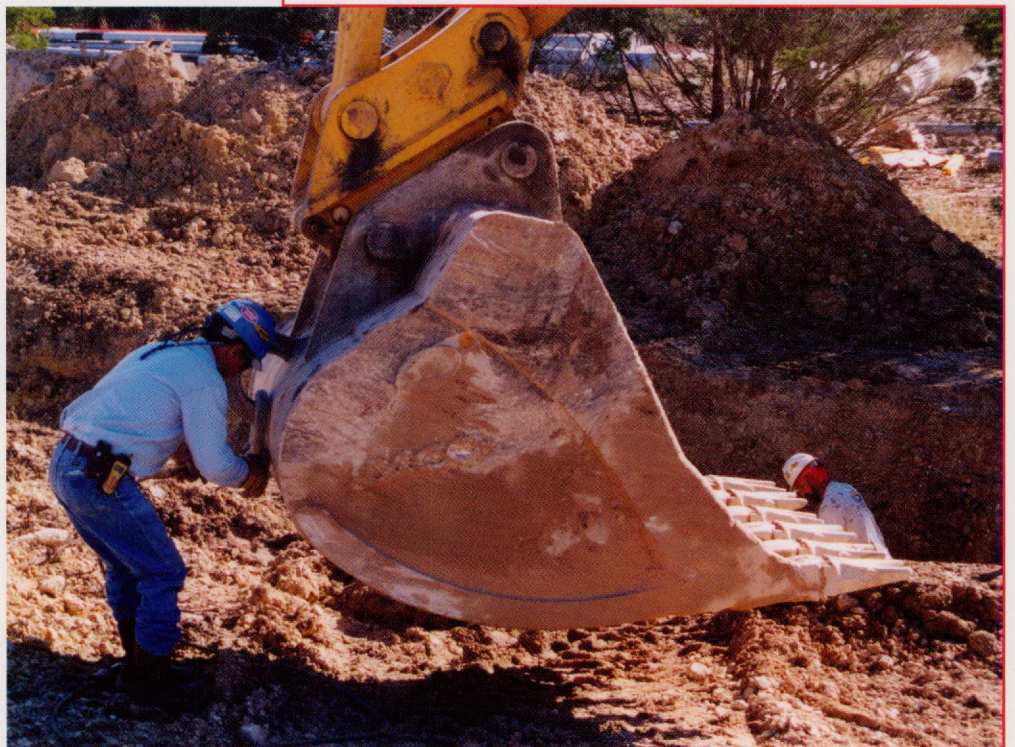
Excavation begins on the treated water delivery line for the water treatment plant, a major component of the Western Canyon Project.
