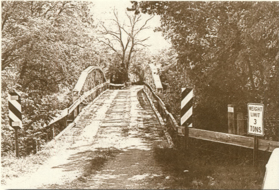
County Road 130 Bridge, Caldwell County, Texas. This old bridge was built in the late 1800's by the Austin Bridge Company of Dallas. It is 59 feet long and is an example of the Warren pony truss construction typical of the period. Photo courtesy of the Caldwell County Genealogical Society.
