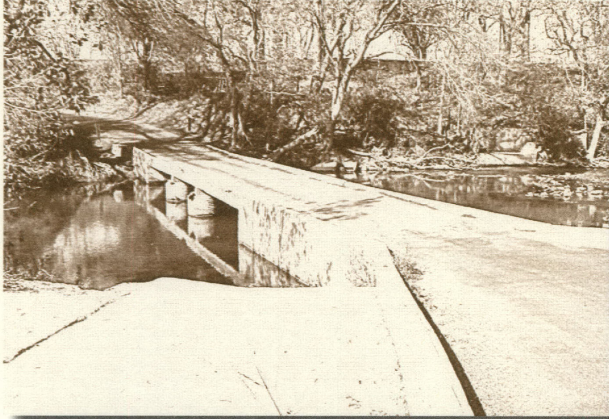
Old Bastrop Highway Bridge at San Marcos, Texas. This bridge is typical of many low-elevation concrete bridges that still carry traffic across rivers and streams in Texas. It is scheduled to be replaced at the beginning of 2007. Photo courtesy of the Hays County Road and Bridge Department.
