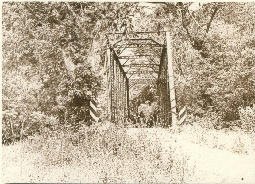
Plum Creek Bridge on County Road 185 east of Clear Fork, Texas. This 119 foot bridge was originally erected across the San Marcos River near Prairie Lea in 1891 by the Groton Iron Bridge Company of Groton, NY. It was later moved to its present location across Plum Creek. Photo courtesy Caldwell Genealogical Society.
