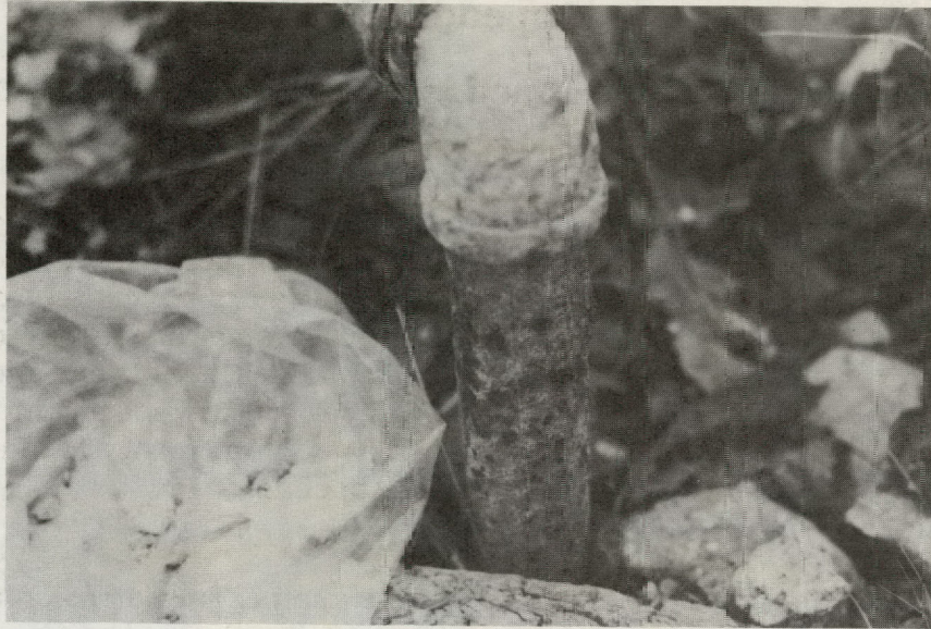
Example of Atmospheric Corrosion
