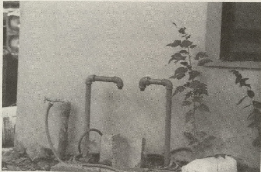
Vacant Meter Loop Properly Plugged
