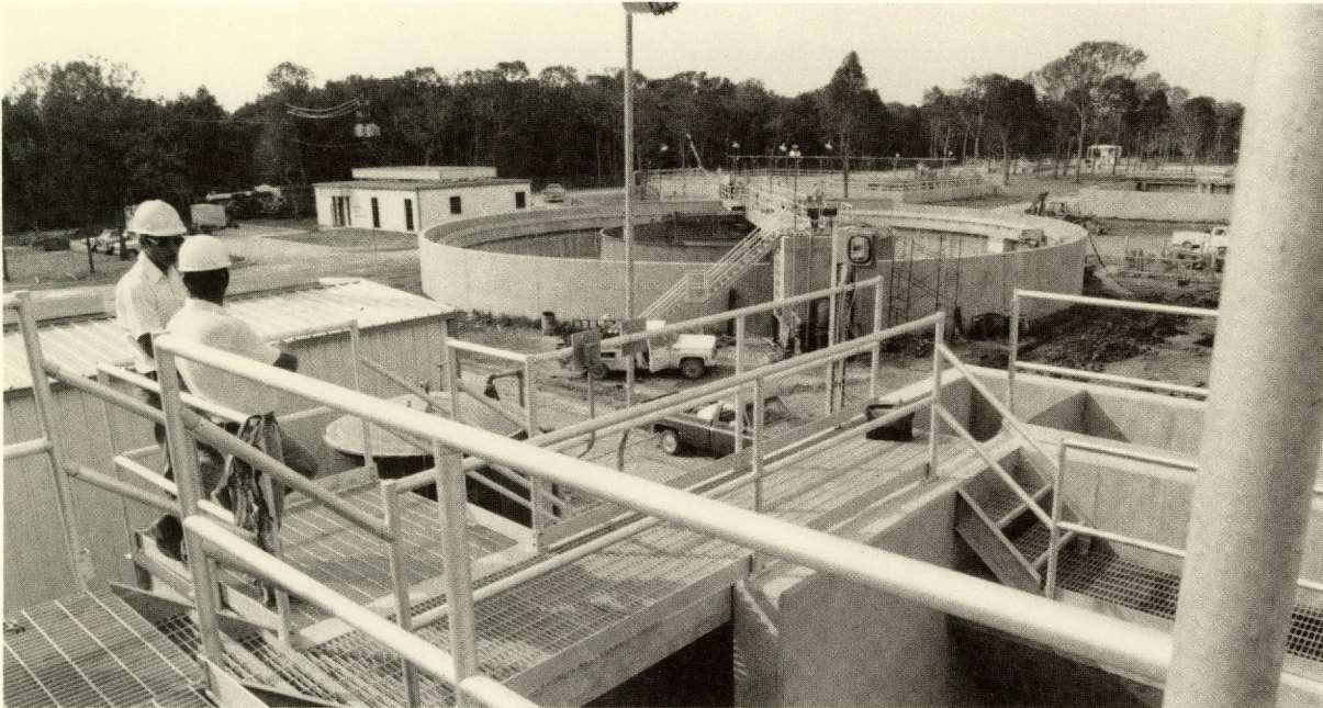
Phase II construction at the Blackhawk Regional Sewage Treatment Facility was completed in 1986 taking capacity from 3.25 mgd. to 9.25 mgd. Blackhawk serves the City of Friendswood, Municipal Utility District 55, MUD 142 (City of Houston) and CDC, Inc.
