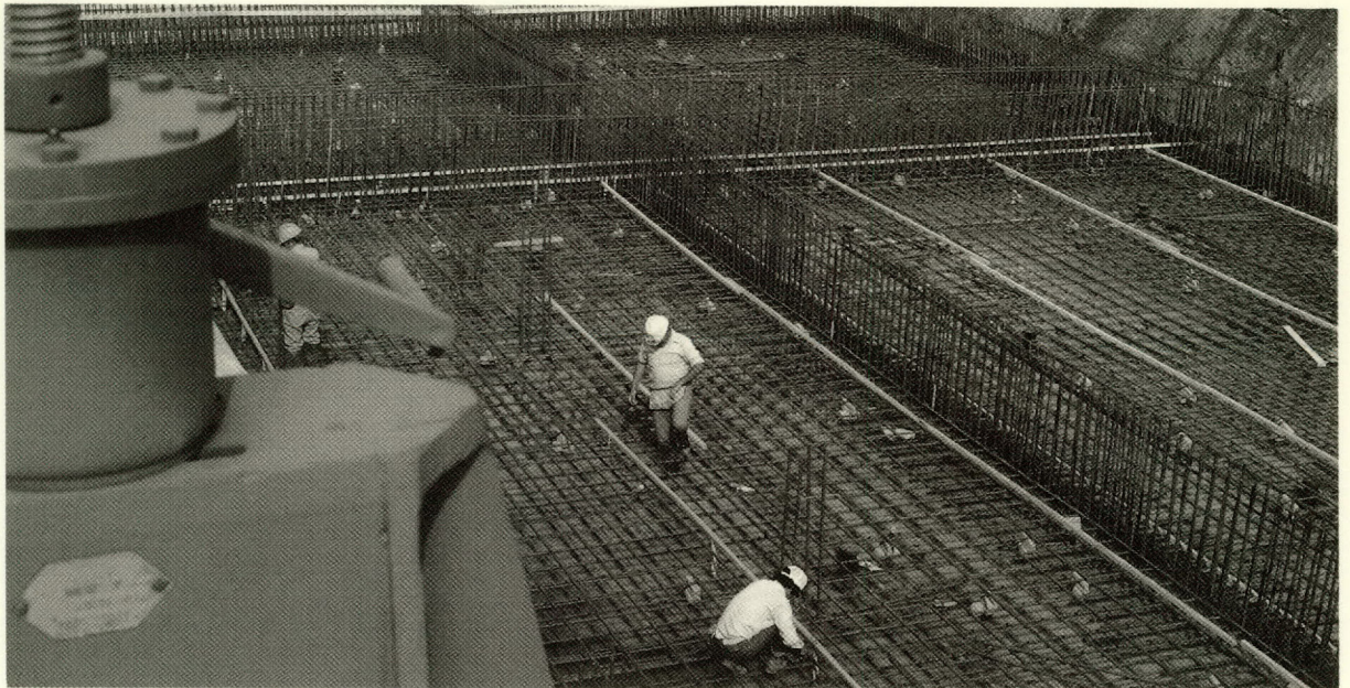
New construction at the Alief Regional Sewage Treatment Plant in 1983 expanded capacity from 1 million gallons per day to 4.0 mgd.
