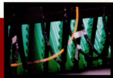
Ultraviolet lights provide the disinfection at the Blackhawk Facility just prior to discharge of treated water to Clear Creek.
