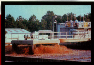
Operators make adjustments atop the headworks. Foreground, surface aerators operate in the initial treatment basin.
