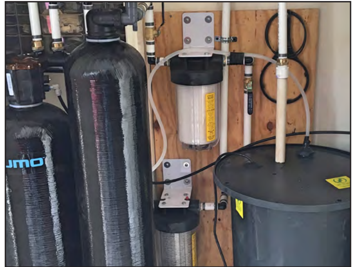
This system collects regeneration backwash from a water softener for use in landscape irrigation.
