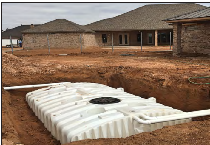
A 2,500 gallon underground storage tank
