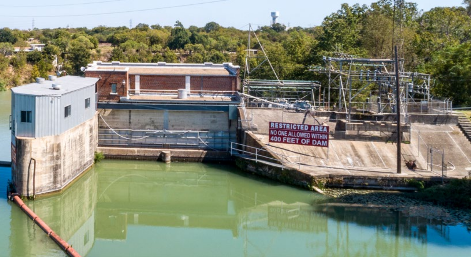
Signage warning of the danger the aging dams pose is installed at all GV lakes dams.
