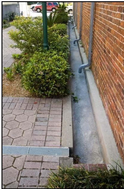
This alley in Valdosta, GA pays special attention to drainage issues while protecting the historic building and hiding the downspouts with plantings placed away from the building. (photo credit: C. Fischetti, Valdosta)
