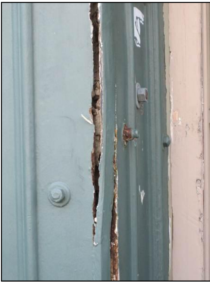
Fig 4 Rust has split the surface of this cast iron column
