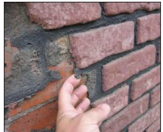
Z-brick, with its false felt, adhesive "mortar," and thin brick, being removed from an original masonry wall.
