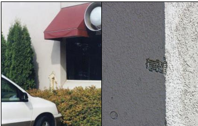
EIFS is highly susceptible to puncturing, especially when installed in close proximity to grade.
