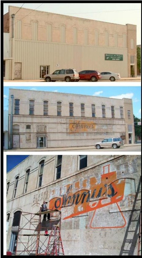
Metal siding has been removed and restoration work is now underway at the Brantley Wright Insurance Building as a result of the Main Street Façade Grant program.
