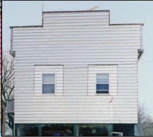
The character-defining cornice, corner boards, trim and even the original windows were all removed to make way for this vinyl siding.
