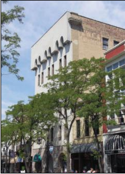
In this case, the EIFS was applied to conceal historic elements of the building, such as this decorative stone cornice.
