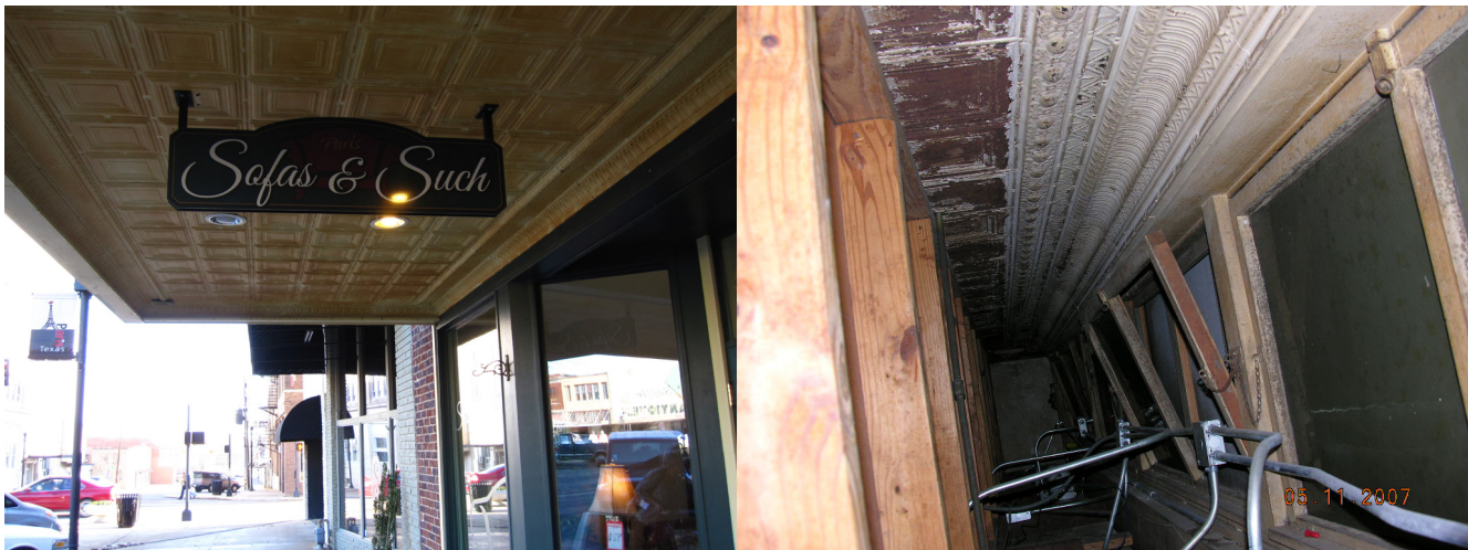
Left: pressed metal soffit on underside of canopy Right: Interior view of encapsulated transom window with pressed metal trim
