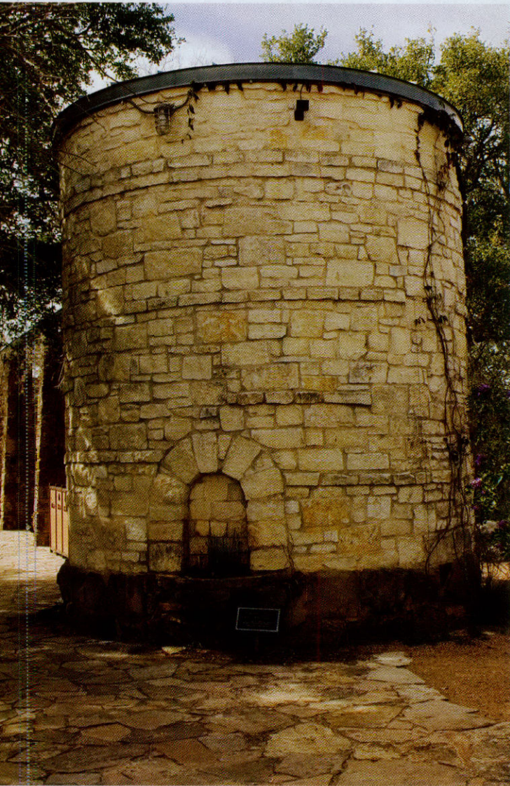
Above: The 12,000-gallon Entry Cistern, one of five that supply 10 to 15 percent of the landscape water at the Lady Bird Johnson Wildflower Center, demonstrates that rainwater collection systems can be beautiful as well as functional.
