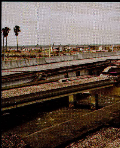
■ (Top right) Game Warden Captain Rod Ousley persuades Angeline Tomkins to leave her Crystal Beach home the morning following the hurricane. (Above) Damage to the Rollover Pass Bridge in Gilchrist. (Right) What wasn't swept away by the tidal surge and subsequent outflow becomes buried.
