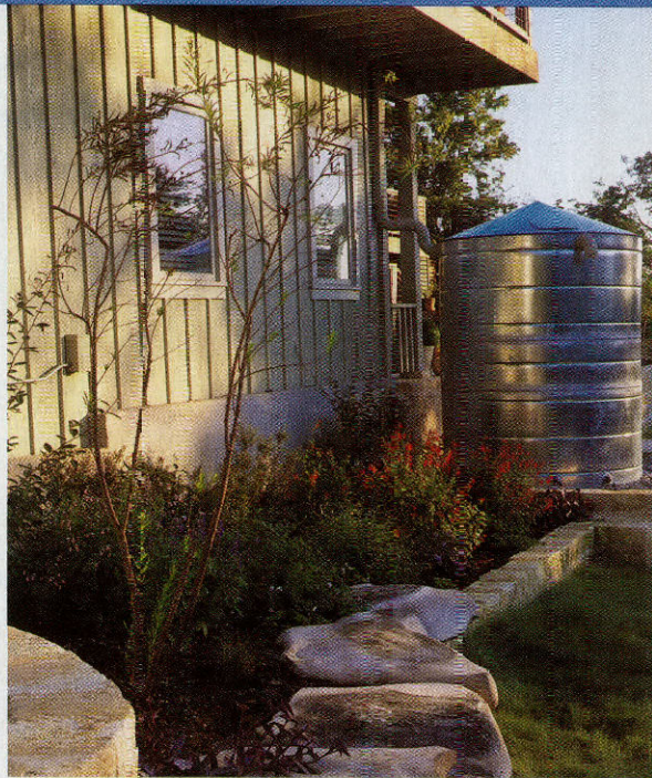
This Austin home has been retrofitted with an eye-pleasing rainwater collecting system.
