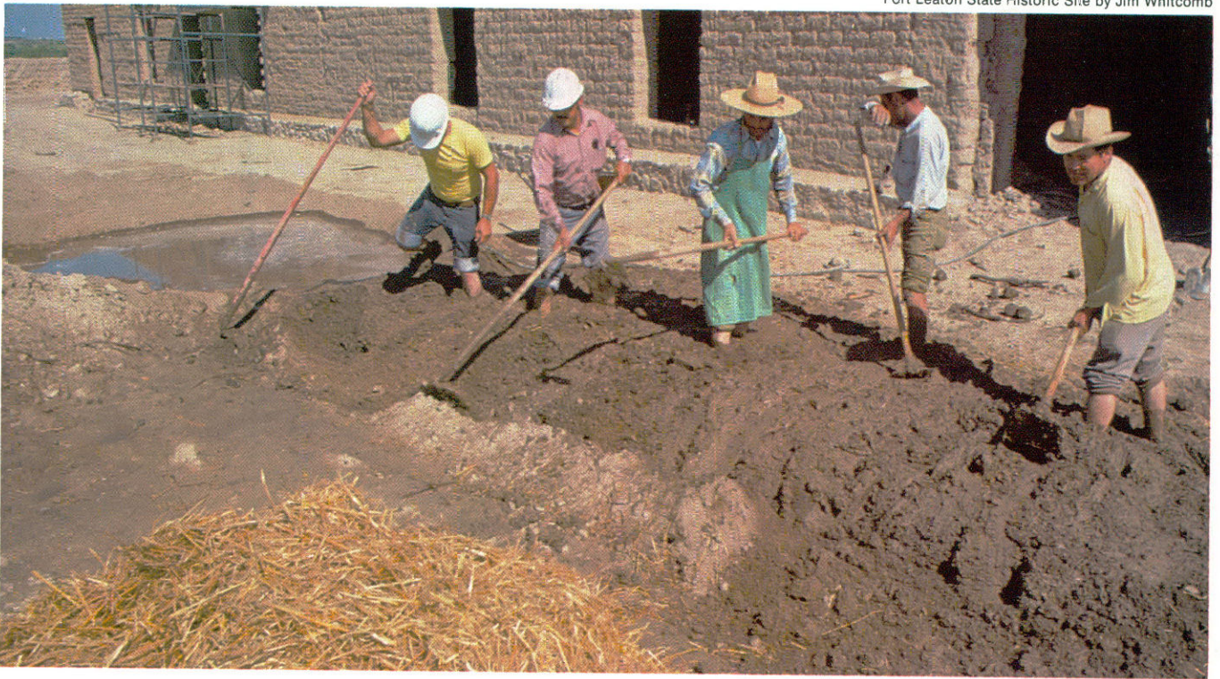
Preserving our historical heritage often involves restoration. Workers at Fort Leaton (above) are mixing hay and mud together until the mixture is suitable for molding the adobe bricks needed for restoration purposes at this historic site. Fishing opportunities abound on state fishing piers, which are especially popular on warm summer nights. Visitors to the nature trails of Palmetto (below) can readily see the unique vegetation preserved by this state park.
