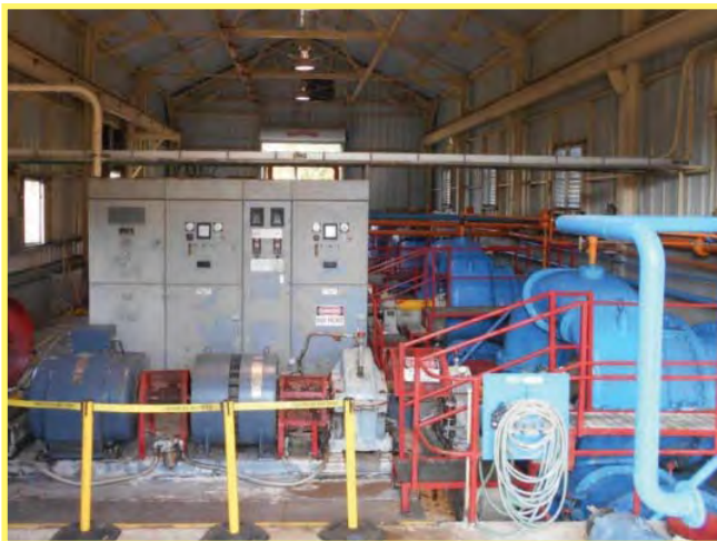
Gulf Coast Pump Station
