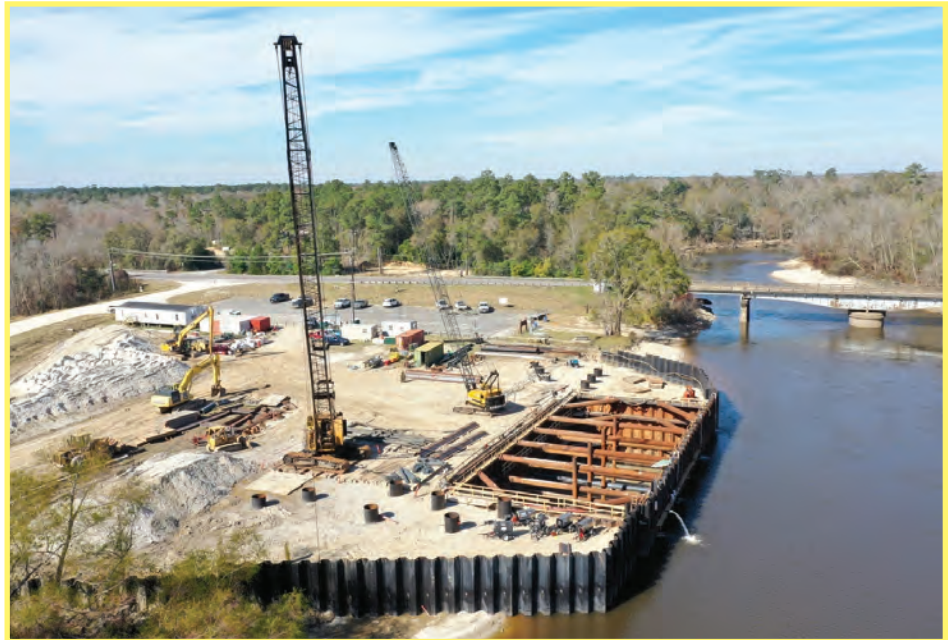
Construction site for the new SRA Gulf Coast Division Pump Station on the Sabine River near State Highway 12
