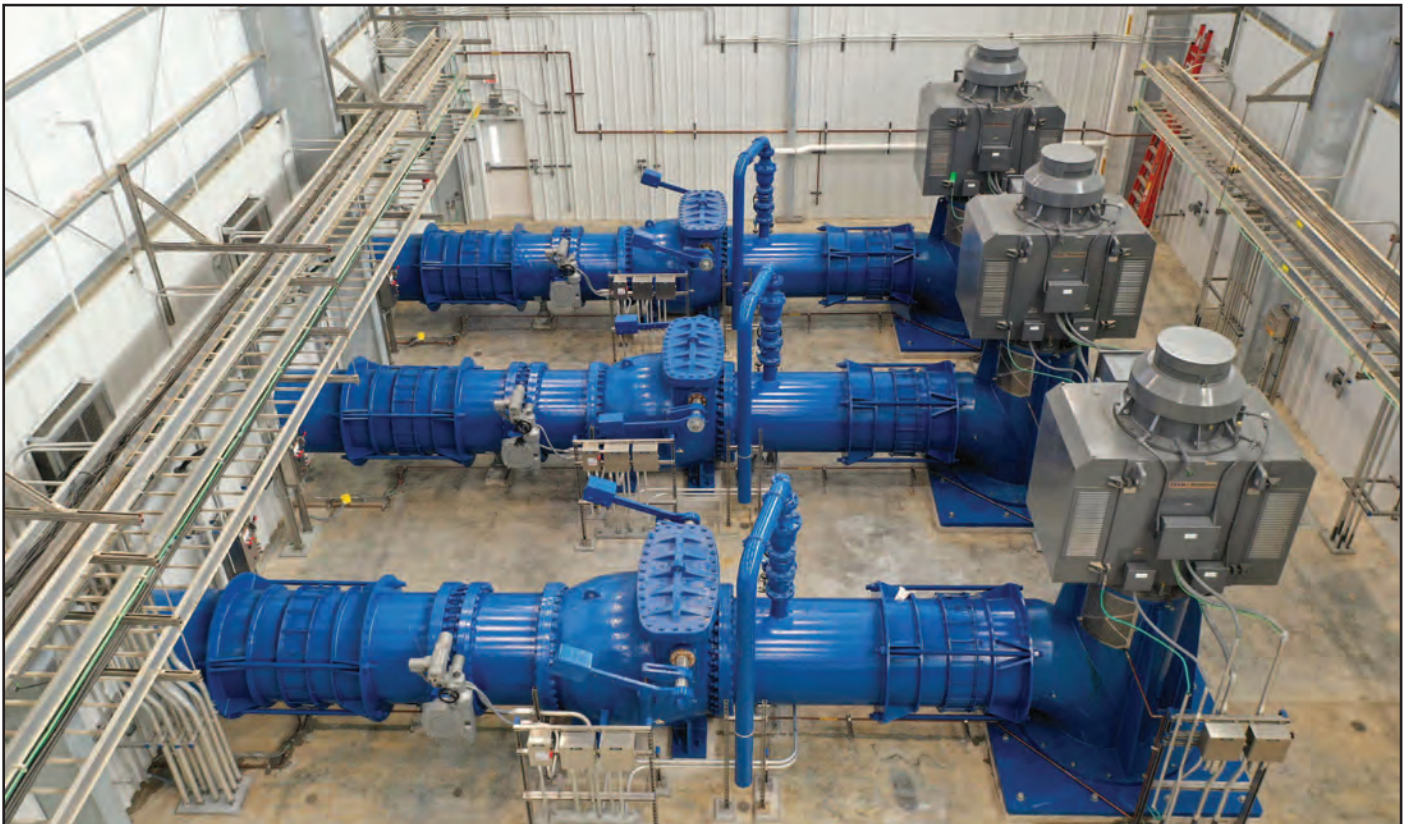
Vertical Turbine Pumps at the New Earl Williams Pump Station
