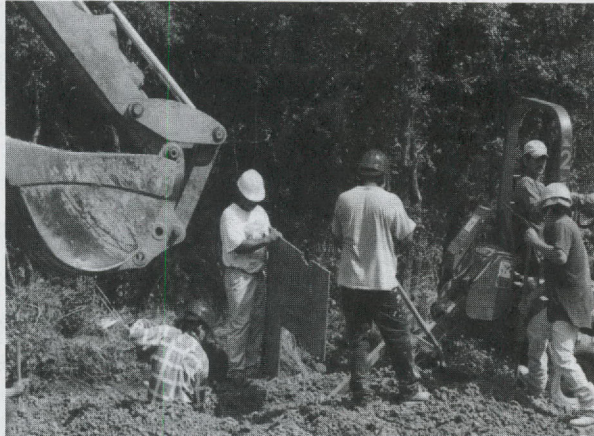
Kennedy Ridge volunteers work on installing their new water and sewer systems.
