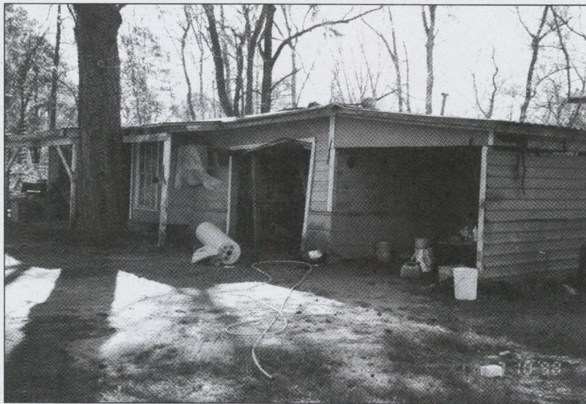
Leon McSwain's wood-frame house was in need of serious repairs he couldn't afford to make when a manufactured housing company and a residential development firm joined forces to make his dream of owning a quality home a reality.
