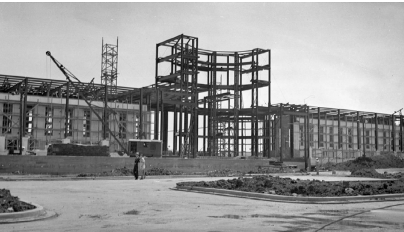
Two months prior to the opening day of the Texas Centennial Exposition, the structural steel frame for the Hall of State was mostly complete and limestone was being placed on the exterior walls of the two side wings.
