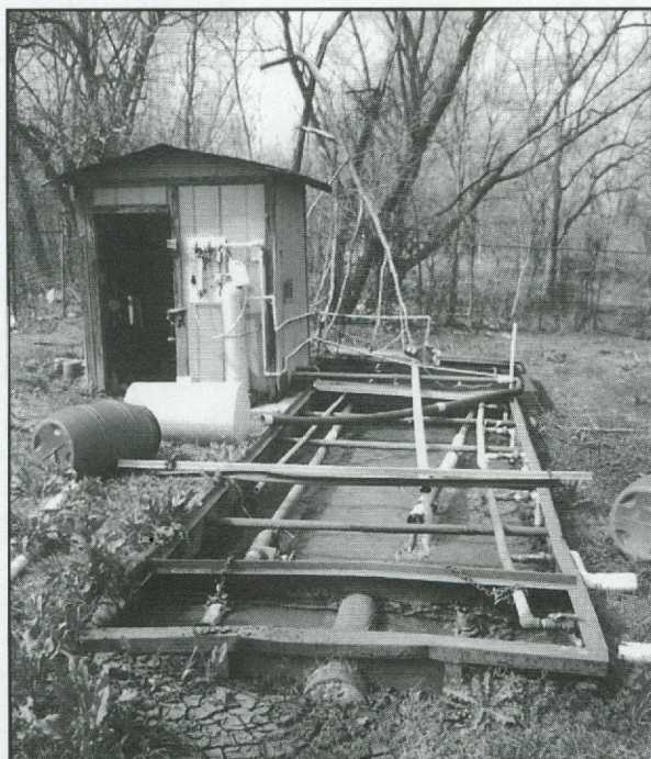
This in-ground sewage treatment plant, which can serve about 50 homes, was one of the more interesting facilities sampled during the project.
