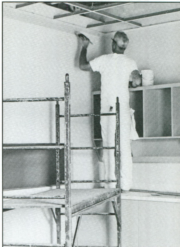
A wing of the Community Services Center was renovated and the college's Child Development Center moved into its spacious new facility in the fall of 1991.
