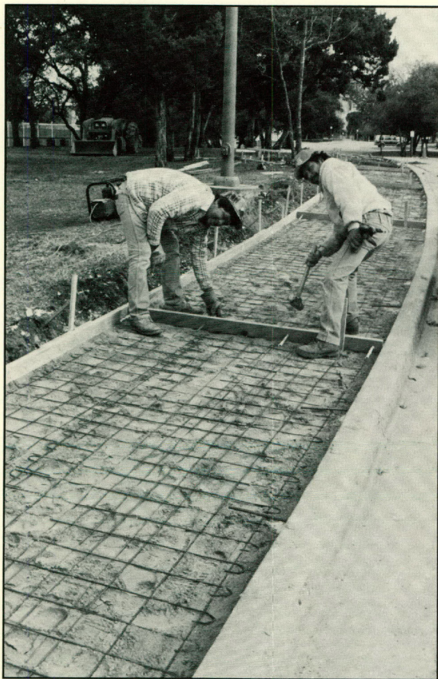
Workers prepare to pour the new sidewalk connecting the Community Services Center and the Health and Physical Education Building.
