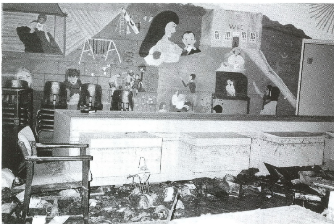
Mud-drenched debris clutters the floor of Project 44's former clinic, and various watermarks on the counter and wall show the levels reached by floodwaters.
