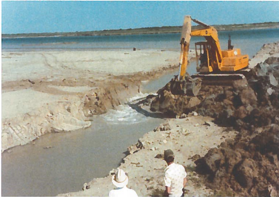
Wally Reed (lower left) watches as Walter Pitt digs a channel connecting the Brownsville Ship Channel with the Bahia Grande in April 1983.
