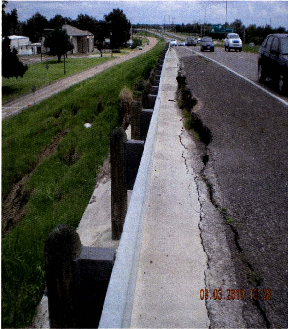
Figure 2.3 Slope failure in the embankment area
