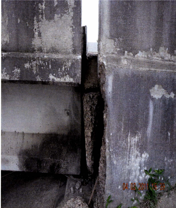
Figure 2.1 Damage in the abutment
