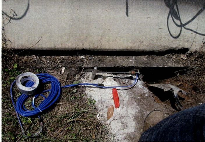
Figure 4.32 Crackmeter installed with the datalogger box
