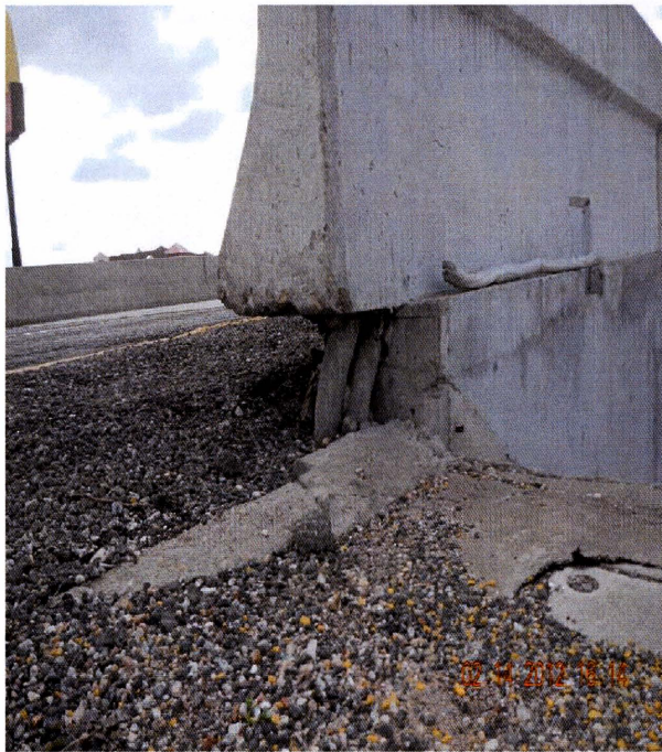
Figure 2.7 Subsidence of embankment material (2)
