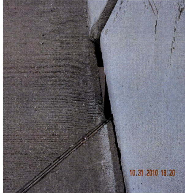
Figure 2.14 Misalignment of traffic rail (2)
