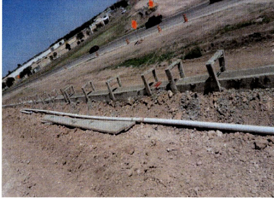
Figure 4.44 Pipes to protect gage cables
