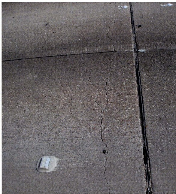
Figure 2.22 Transverse cracks due to voids
