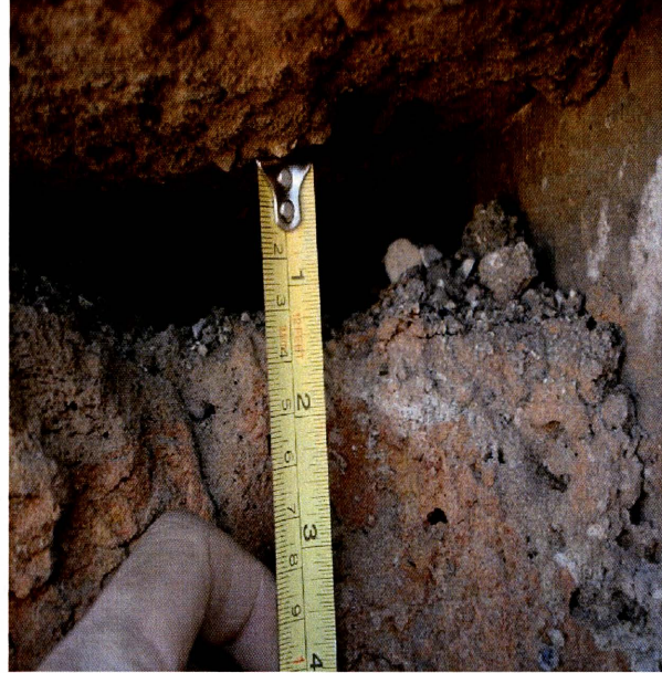
Figure 2.20 Void under bridge approach slab
