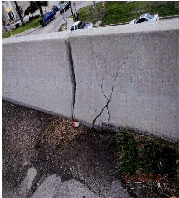
Figure 2.8 Damage in traffic rail
