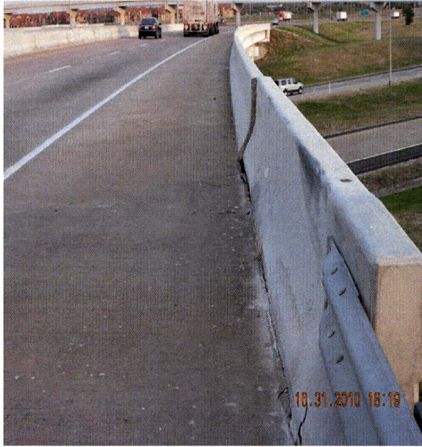
Figure 2.13 Misalignment of traffic rail (1)
