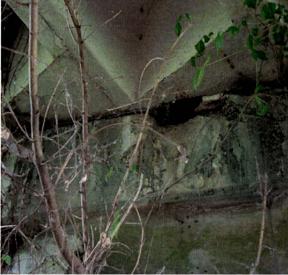
Figure 2.11 Damage in bent cap
