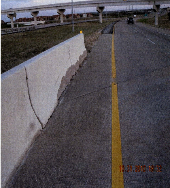
Figure 2.15 Damage in traffic rail
