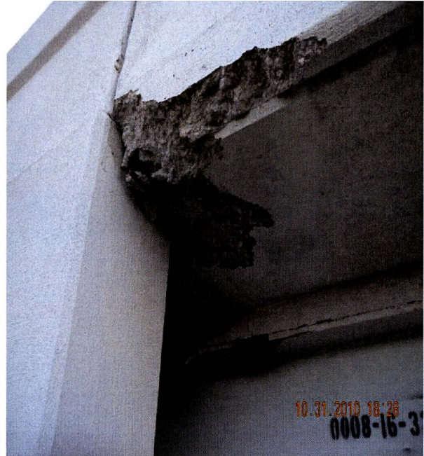
Figure 2.16 Damage in the bridge superstructure
