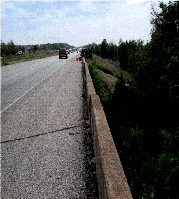
Figure 2.9 Misalignment of the traffic rails
