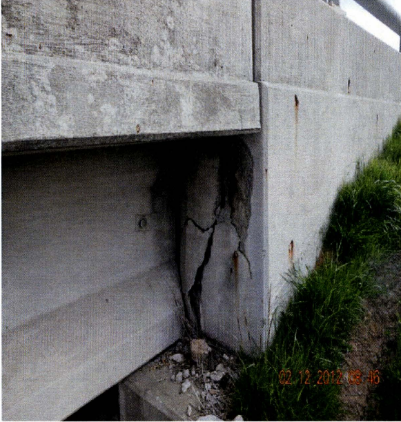
Figure 2.17 Damages in abutment
