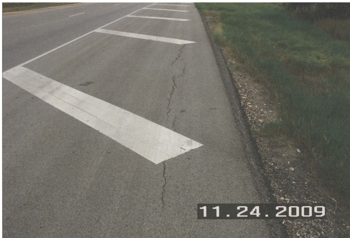
Figure 8.3: Cracking along pavement shoulder in CAM section on Loop 20, Laredo
