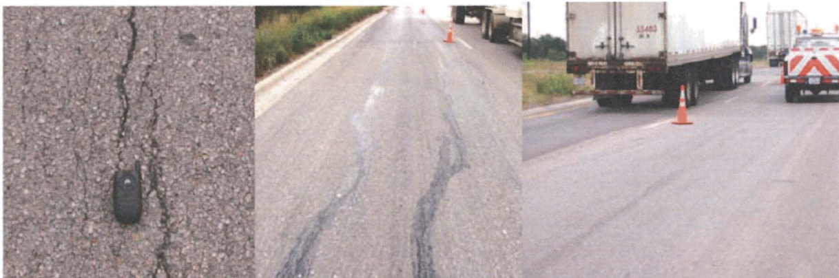
Figure 2.8: Shrinkage cracking distress on FM 734
