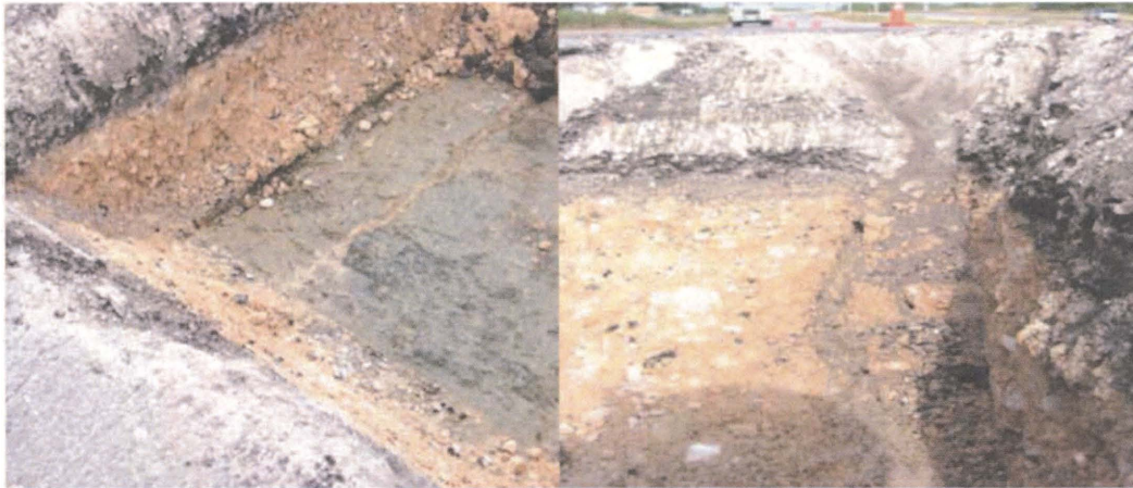
Figure 2.9: Reflective shrinkage cracking seen in test pit
