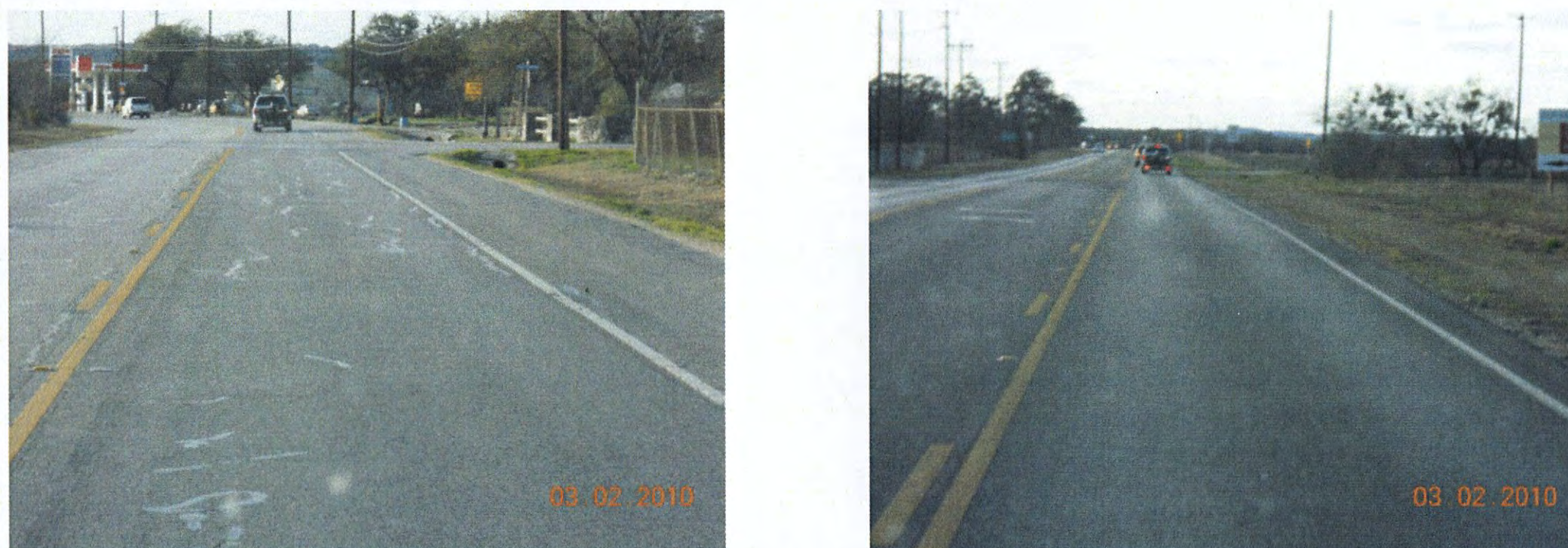
Figure 4.11. Surface Condition Showing Rutting and Cracking in the Wheel Path at the Control (left) and Distress-Free at the Reconstructed (right) Sections.
