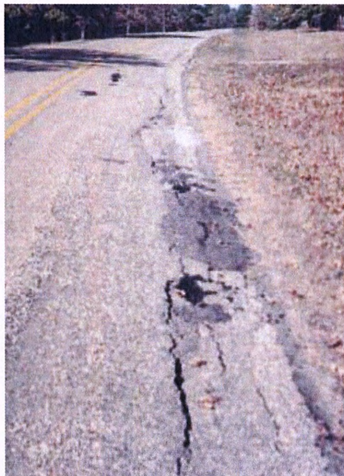
Figure 2.1. Longitudinal cracking and failure (Sebesta 2005).
