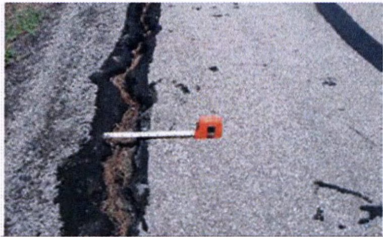
(a) Edge breaks due to loss of adhesion
