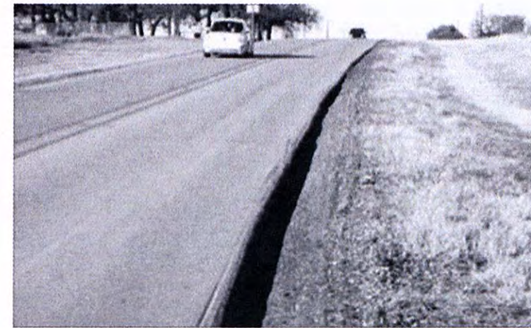
(b) Edge drop-off due to erosion
