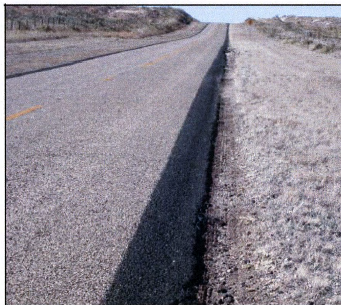
Figure 2.8. Pavement edge drop-off.
