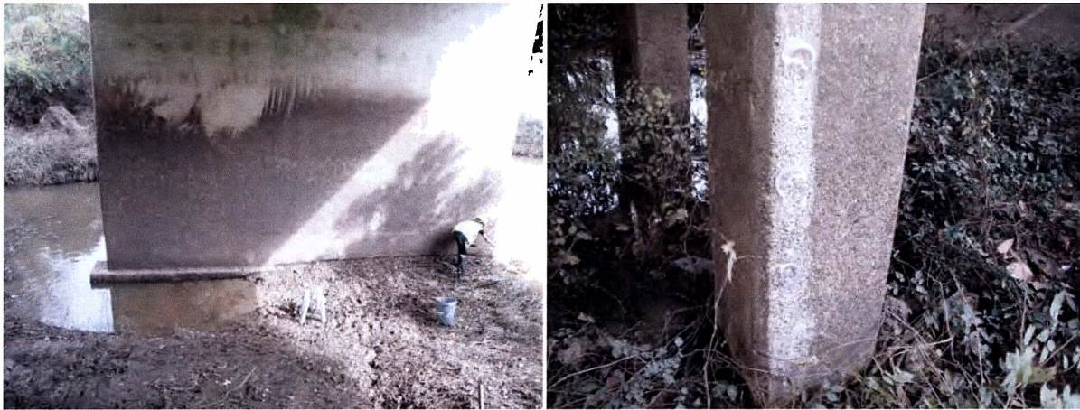
Figure B. 2. Overview of Bridge Deterioration (Bridge 2)
