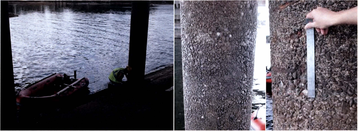
Figure B. 6. Overview of Bridge Deterioration (Bridge 6).
