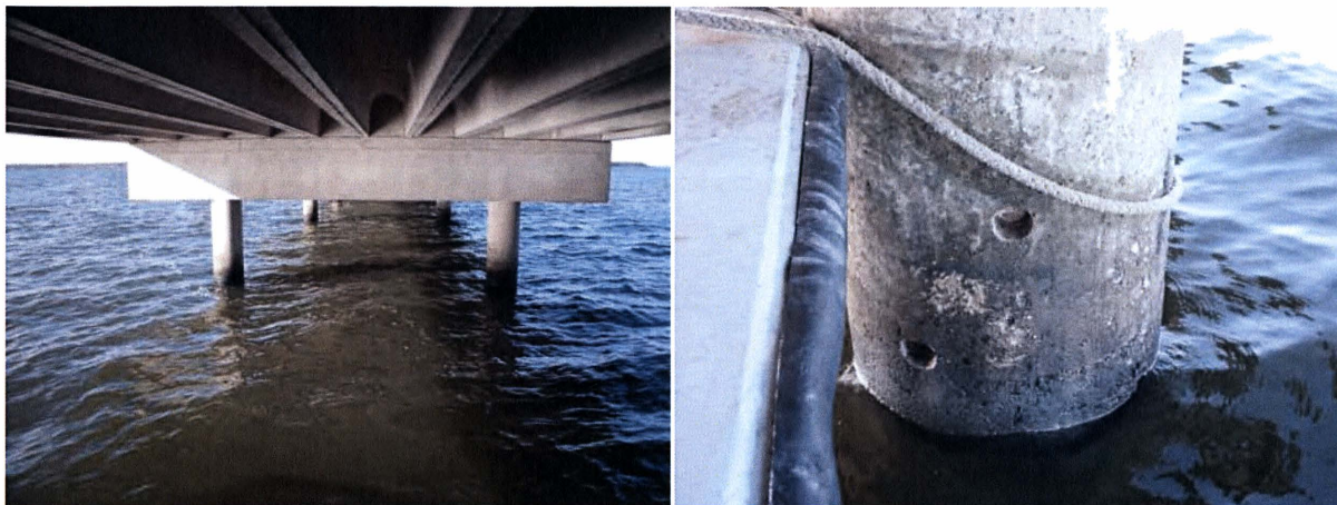
Figure B. 3. Overview of Bridge Deterioration (Bridge 3).
