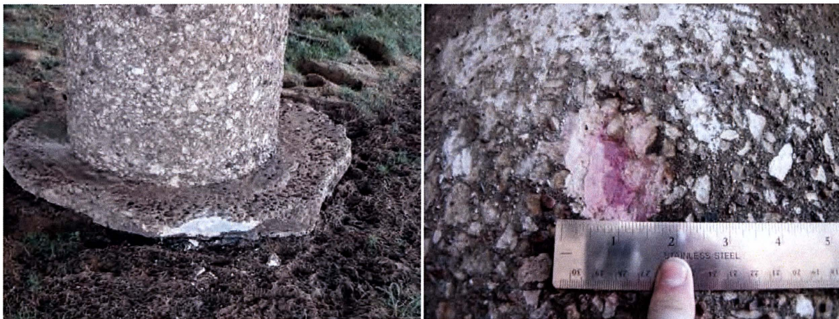
Figure B. 7. Overview of Bridge Deterioration (Bridge 7).
