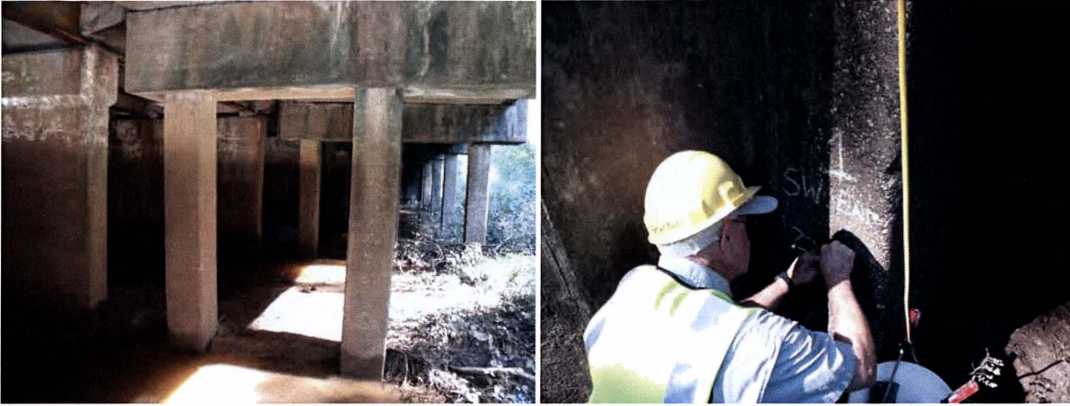
Figure B. 1. Overview of Bridge Deterioration (Bridge 1).
