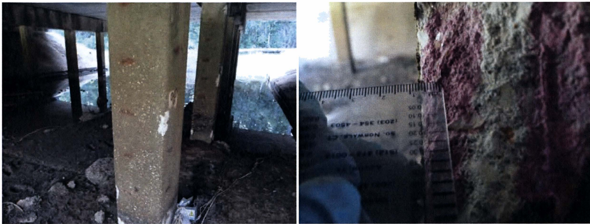
Figure B. 10. Overview of Bridge Deterioration (Bridge 10).
