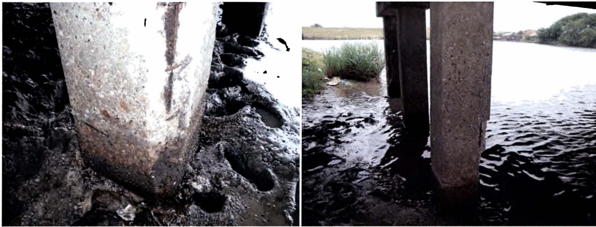
Figure B. 4. Overview of Bridge Deterioration (Bridge 4).
