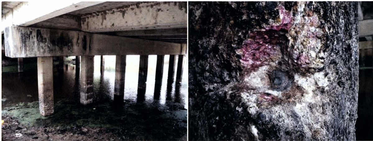
Figure B. 8. Overview of Bridge Deterioration (Bridge 8).
