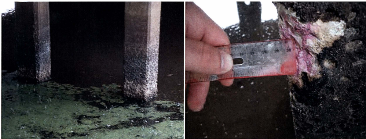
Figure B. 9. Overview of Bridge Deterioration (Bridge 9).
