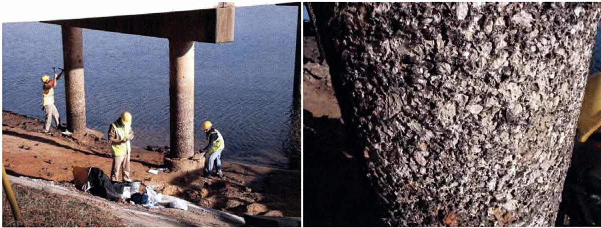
Figure B. 5. Overview of Bridge Deterioration (Bridge 5).
