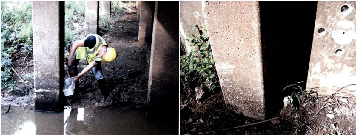
Figure B. 13. Overview of Bridge Deterioration (Bridge 1R).
