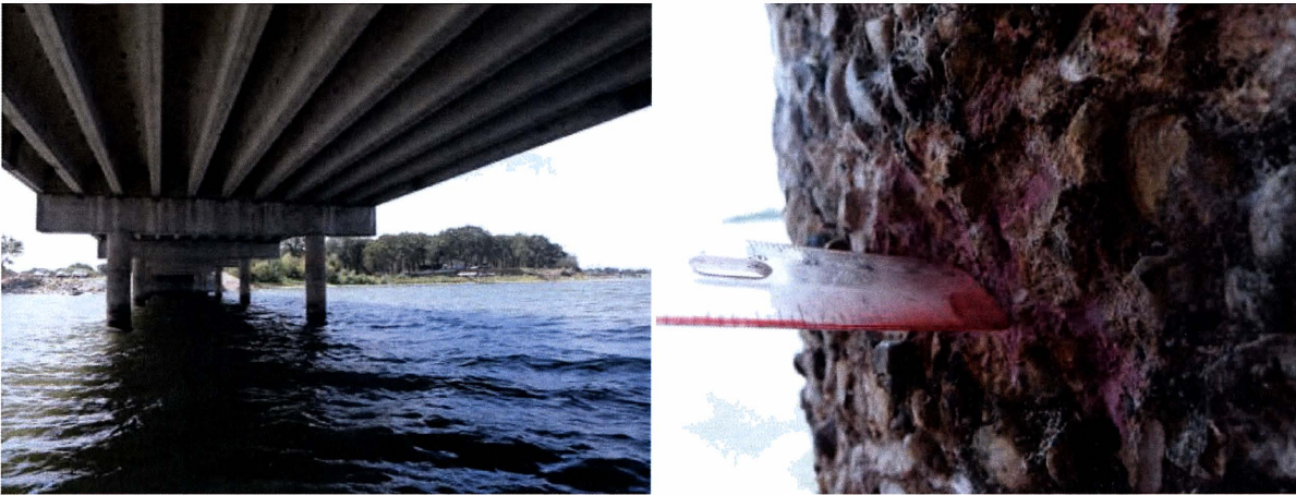
Figure B. 12. Overview of Bridge Deterioration (Bridge 12).
