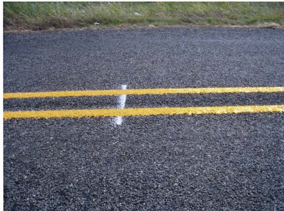
Figure 10. FM 1680 Road Surface with Marking.
