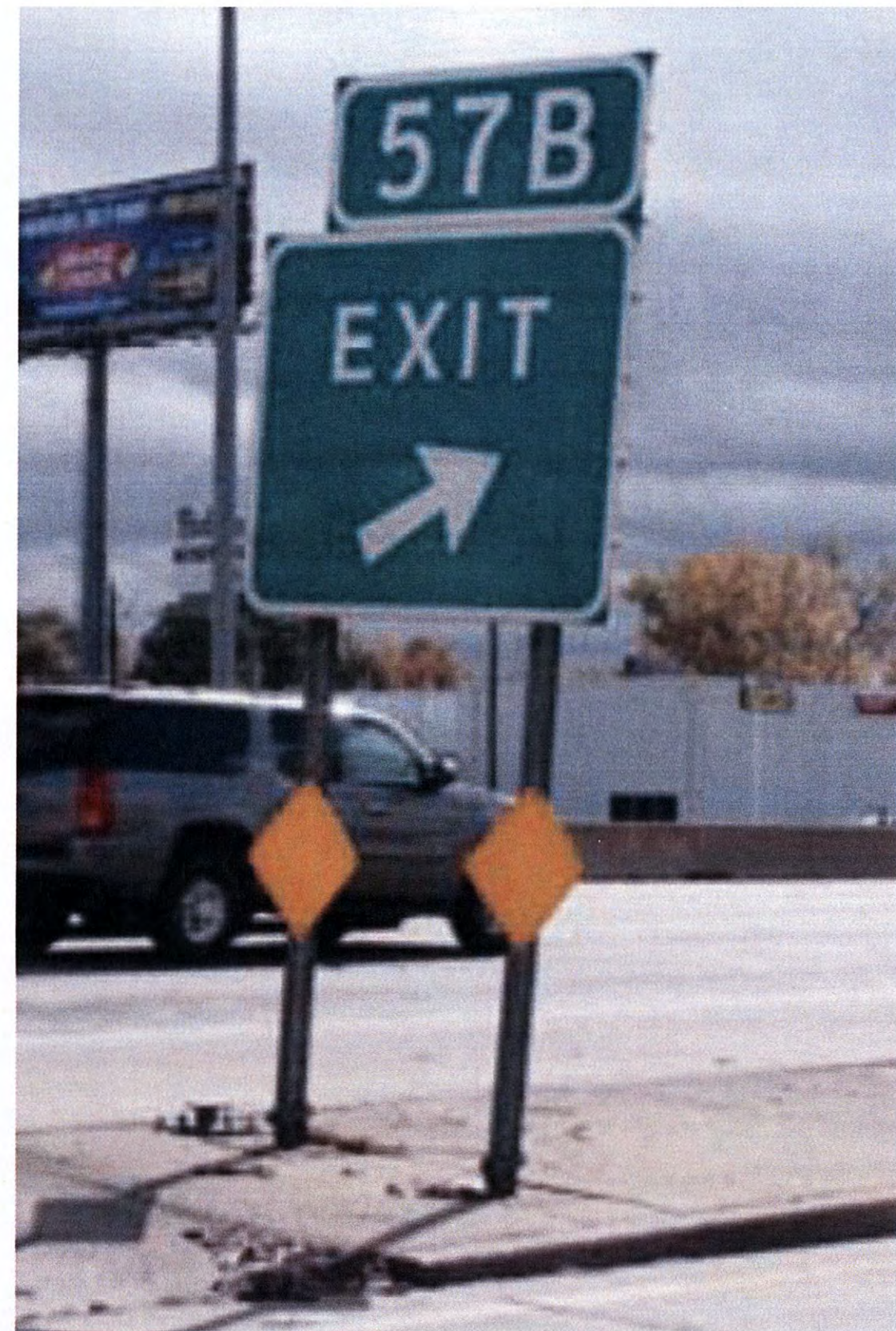
Figure 24. Reflective Object Markers on Sign Posts.
