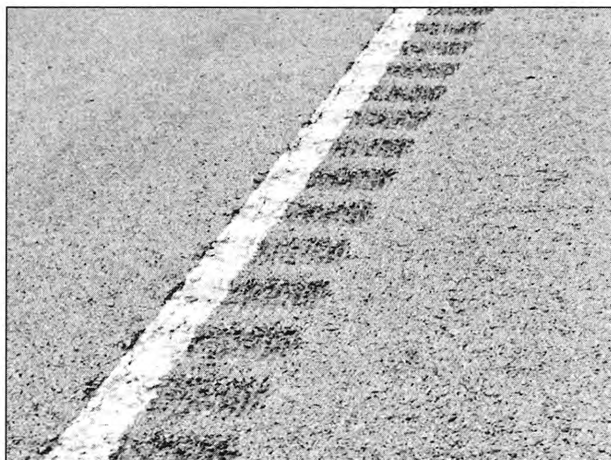
Figure 5. Rumble Stripe Pavement Marking.
