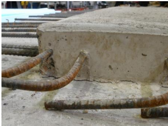
(a) Cracking between Stage I and II
