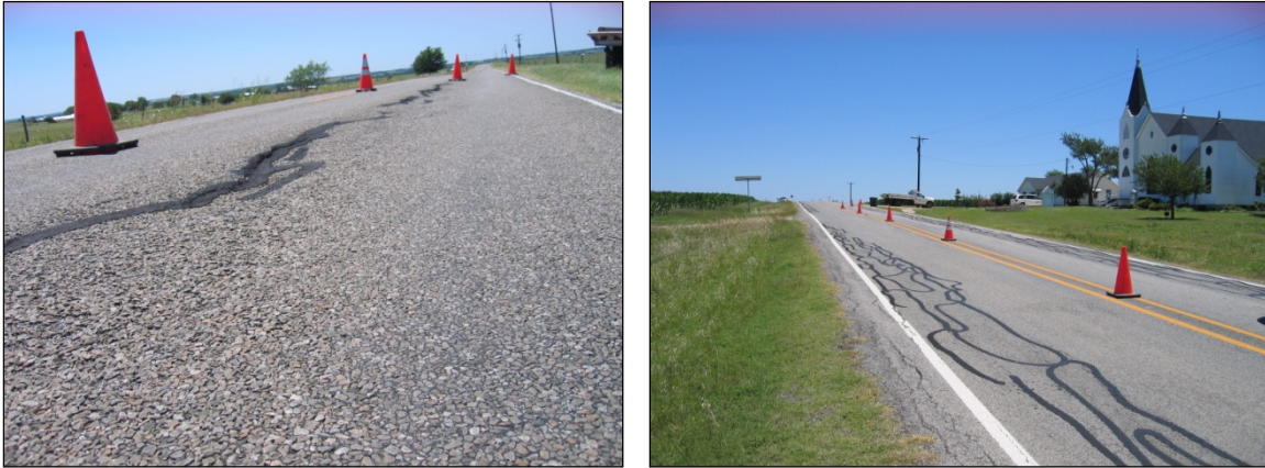
Figure 4.6. Pavement Distress on FM 112.
