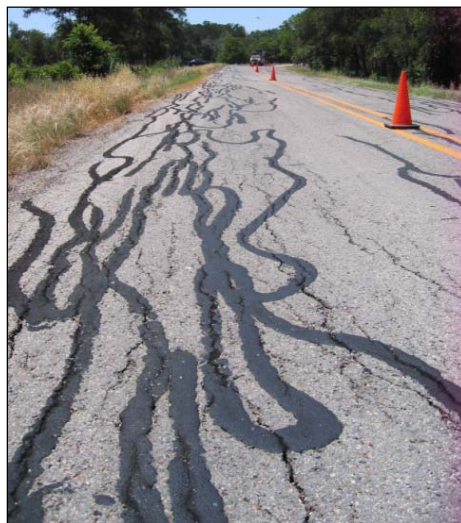
Figure 4.7. Longitudinal Cracking on FM 112.
