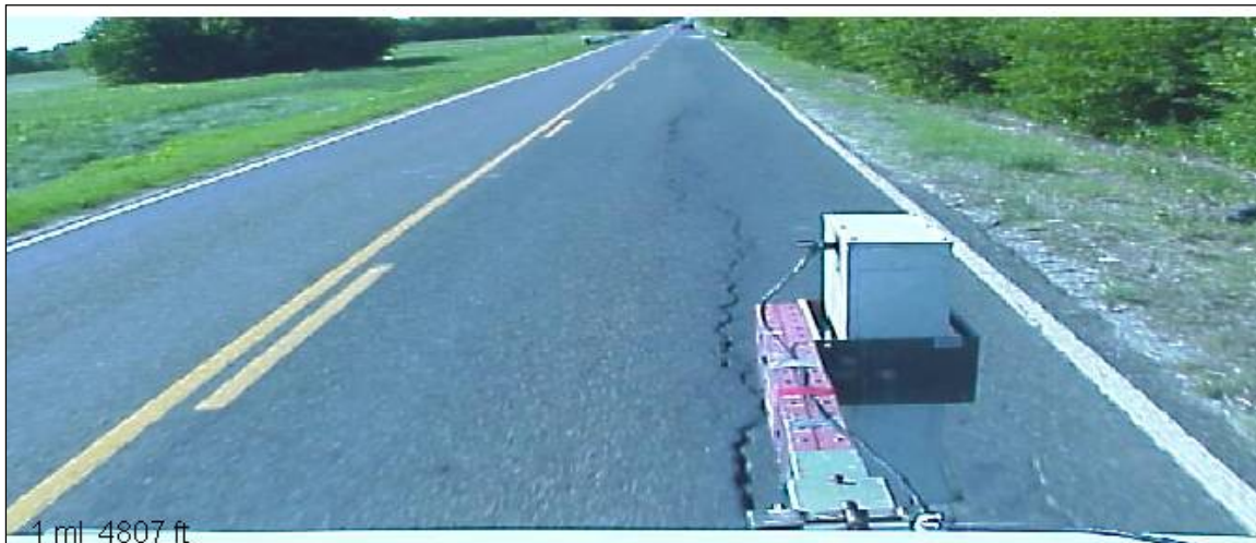
Figure 6.1. Pavement Distress on Business (US) 289.
