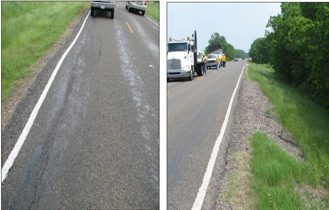
Figure 7.1. Typical Edge Failure on FM 148.
