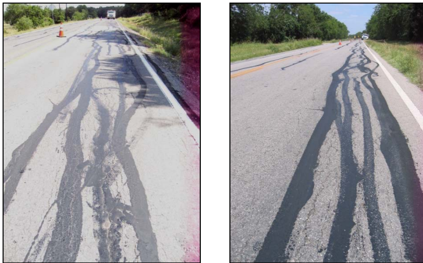
Figure 5.1. Typical Distress on FM 969.
