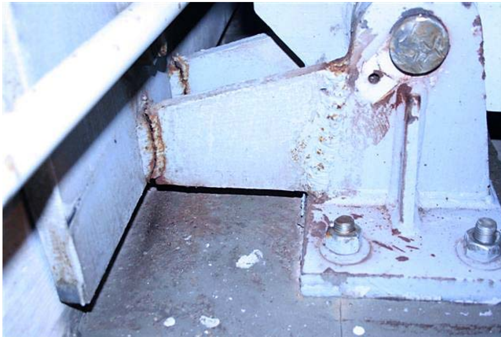
Figure 29. Photograph of Cracked Bearing Assembly.
