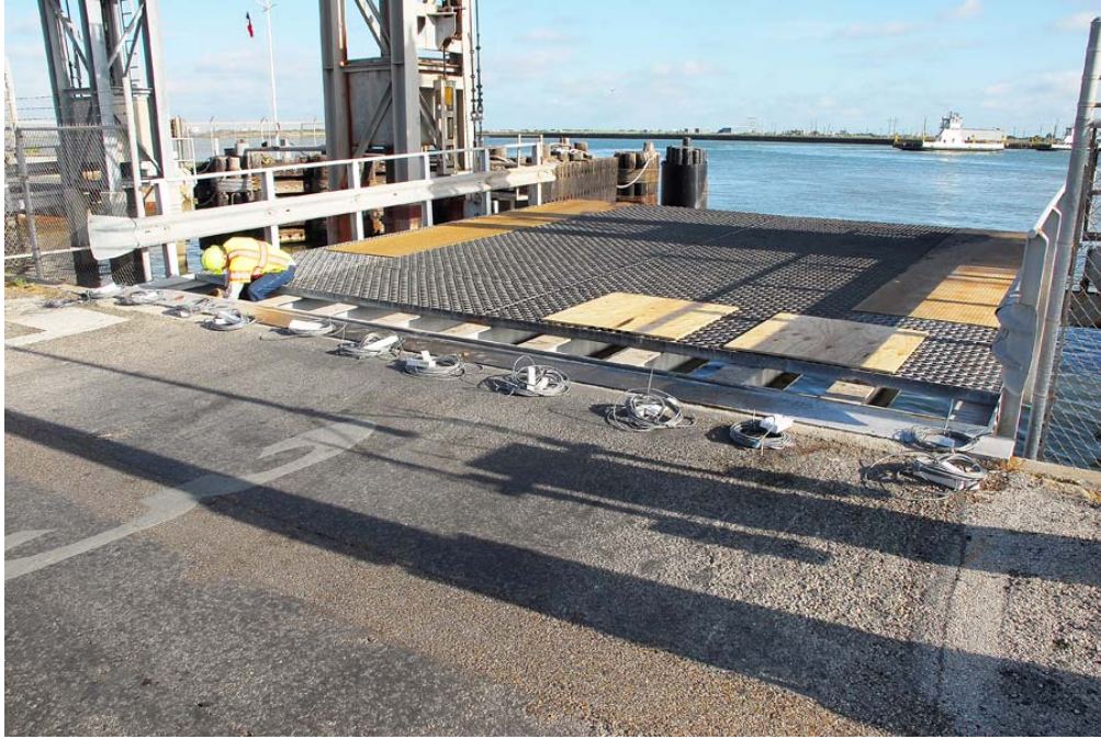
Figure 32. Photograph of Instruments with Cables Attached Ready to be Installed.
