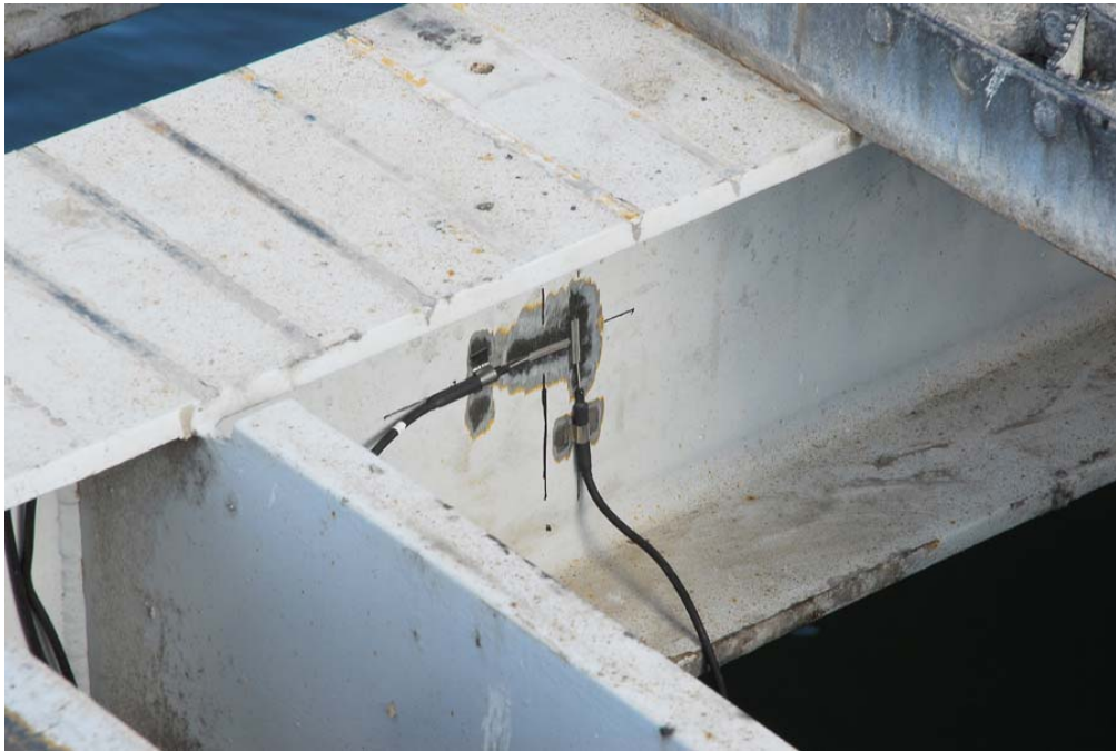
Figure 35. Photograph of Typical Sensor as Installed.
