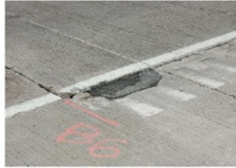
Areas to be repaired prior to BCO placement marked with spray paint
