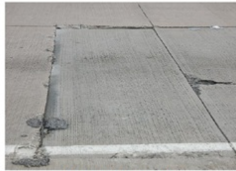
Damaged PCC patch
