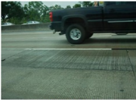
PCC patch with spall
