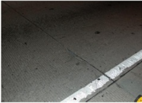
Spall at joint
