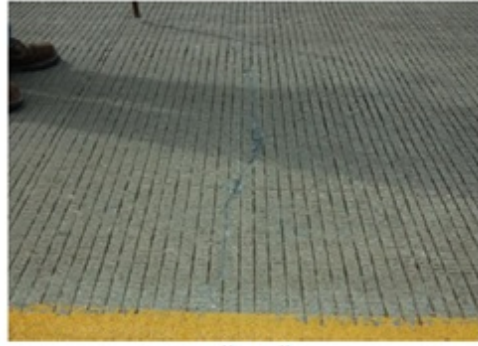
Small spalls 1989-1990 Experimental sections (EB)
