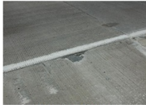
Shoulder joint damage
