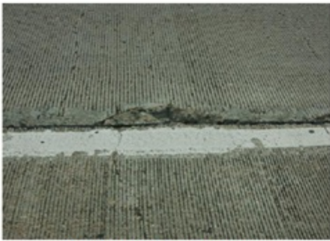
Longitudinal joint damage
