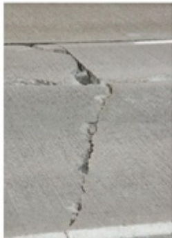
Wide crack and punchout
