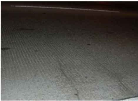
Typical transverse cracks
