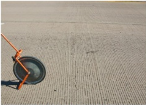
Typical transverse crack
