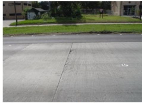
Patch with spall
