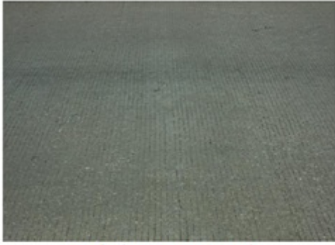
Typical transverse crack 1989-1990 Experimental sections (EB)
