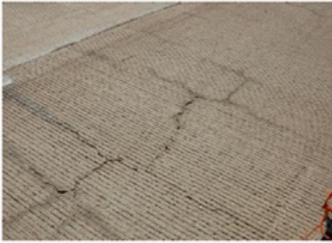
Transverse and longitudinal cracks (area of potential punchout)
