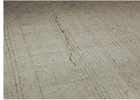
Transverse and longitudinal cracks
