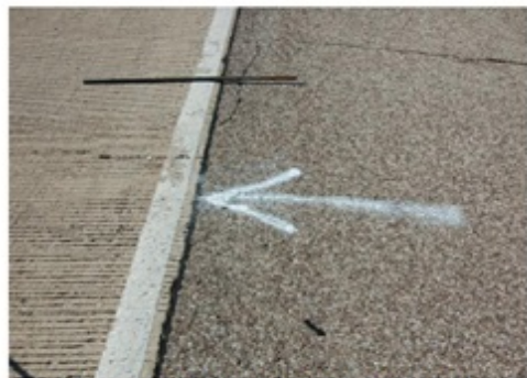
Delaminated area (edge of lane)
