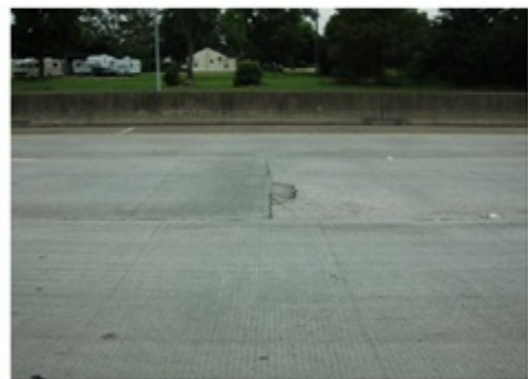
Patch with Failure
