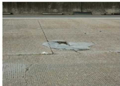
AC patch with failure
