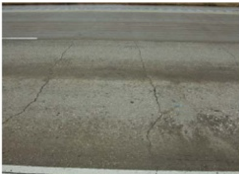
Picture 3 Transverse cracks
