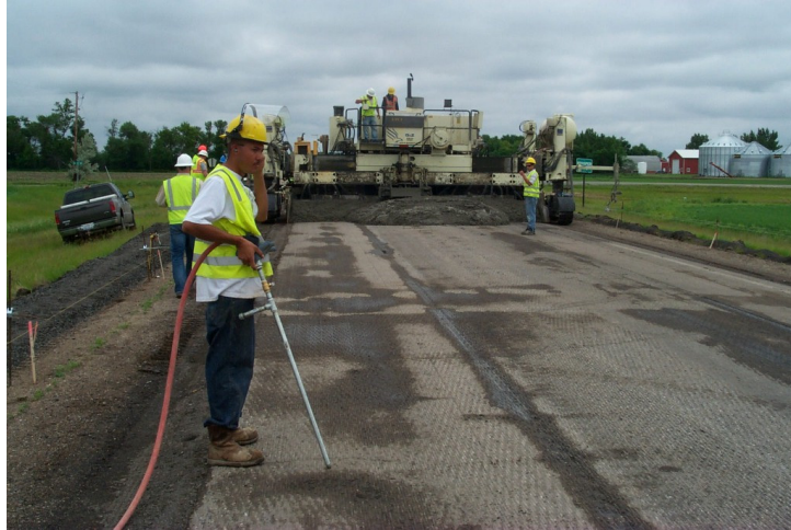
Figure 7.5: Use of an air hose to clean the surface and spread pooled water just ahead of the paver
