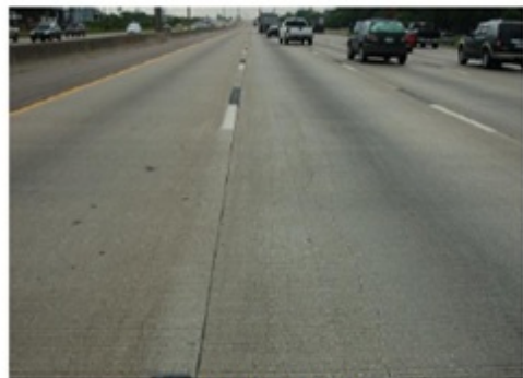
Longitudinal crack 1989-1990 Experimental sections (EB)
