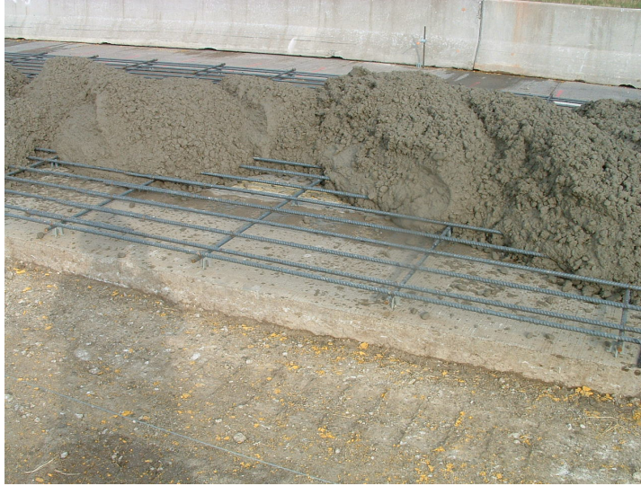
Figure 3.11: Dried surface around concrete
