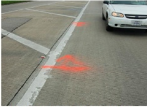
Delaminated area, next to exit ramp 1983 Experimental sections
