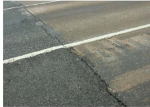
Picture 2 RM 51. Joint between ACP and whitetopping overlay
