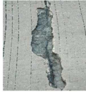
Fibers seen in spall
