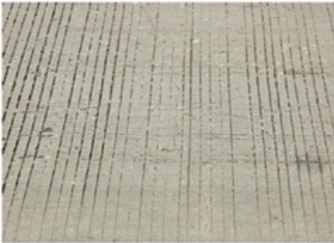
Typical transverse crack
