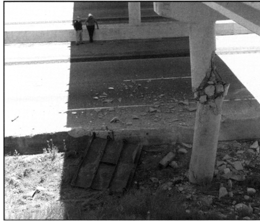
A 39-ton steel girder, when it collided with this I-20 bridge on April 16 near Kilgore left this column looking like a broken piece of chalk.
