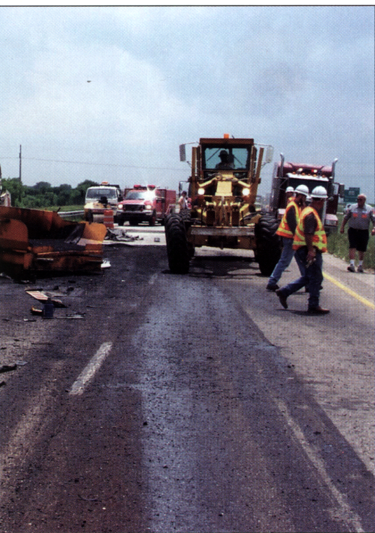
Debris litters the roadway after a car-hauling truck smashed into a work-zone. Two TxDOT inspectors jumped a guardrail to avoid the oncoming truck.
