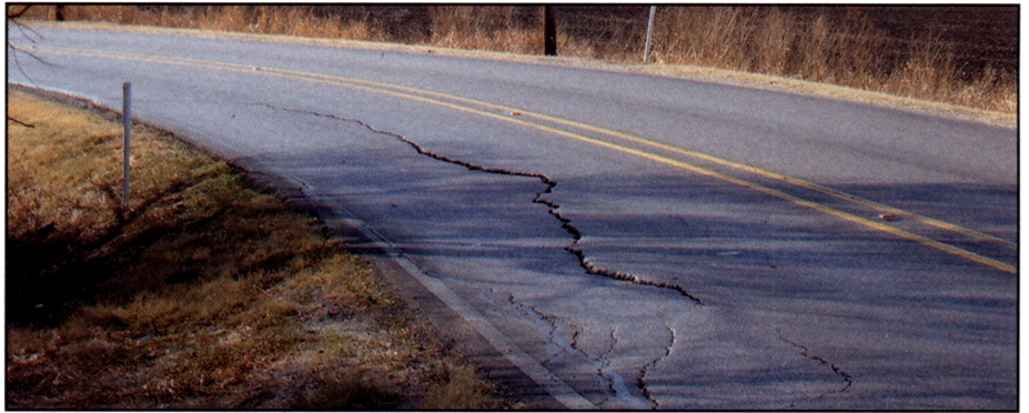
Effects of drought degrade road surfaces.
