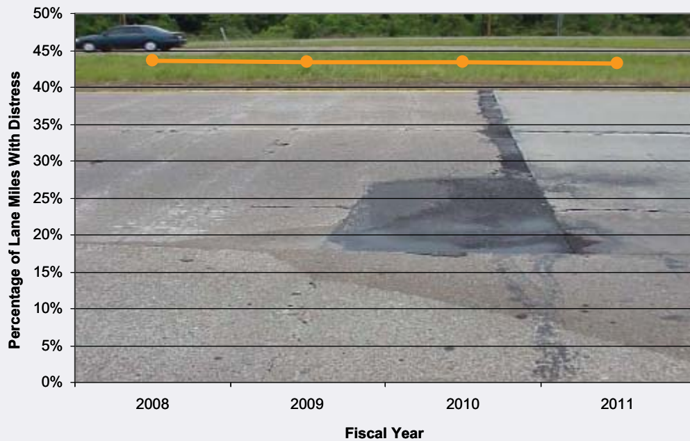
JCP Failures (rated), FY 2008-2011
