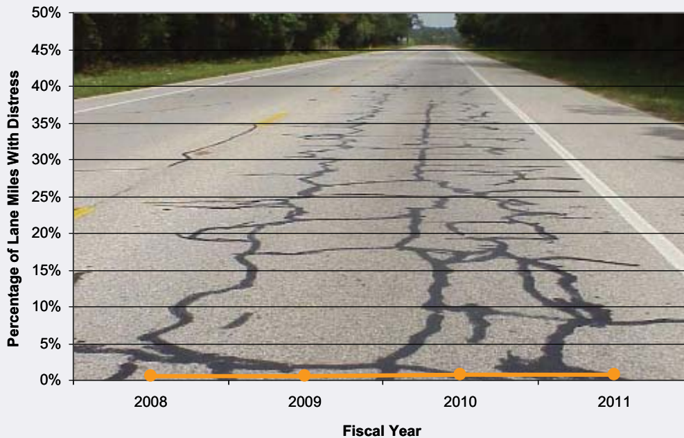
ACP Block Cracking (rated), FY 2008-2011
