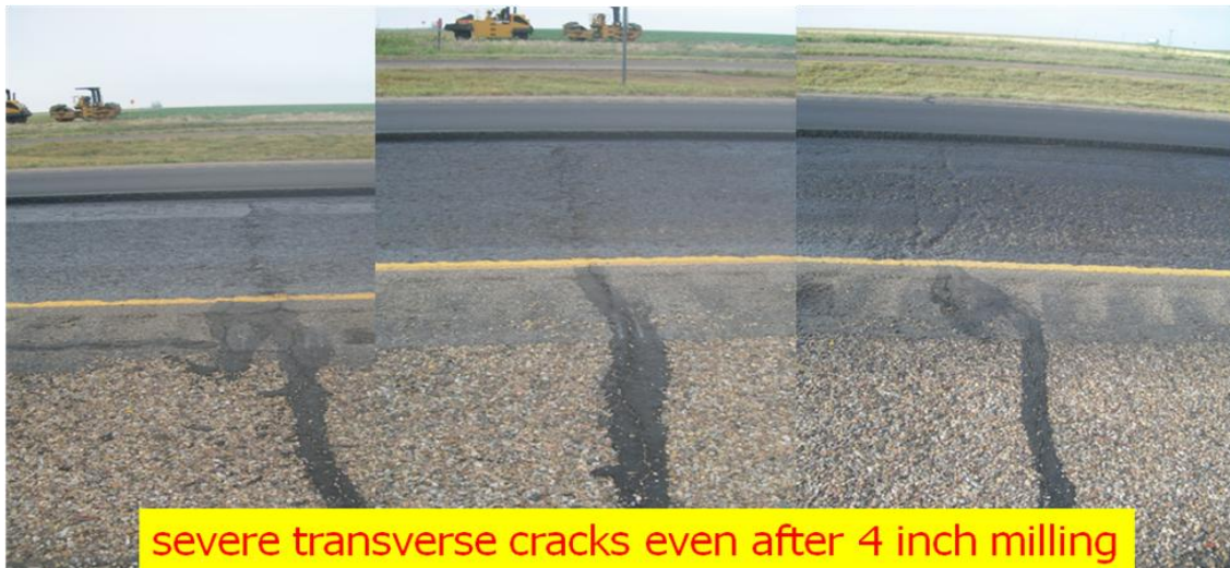
Figure 17. Existing Pavement Conditions of IH40 after Milling.
