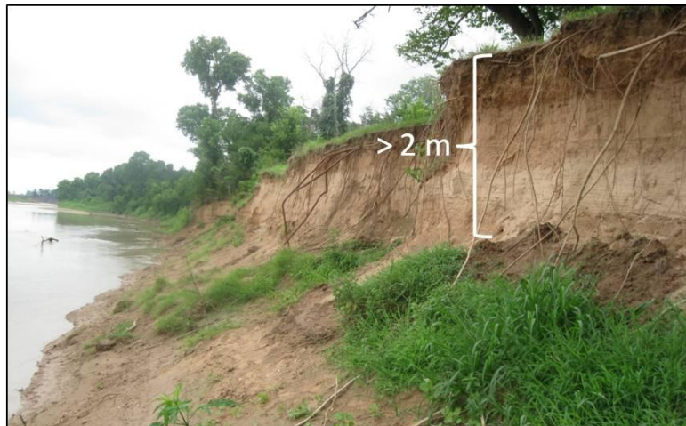
Figure 20. Inner bank with slump toe. The vegetation is not extensive along the bank and the area has experienced deforestation since the 1995 time frame.
