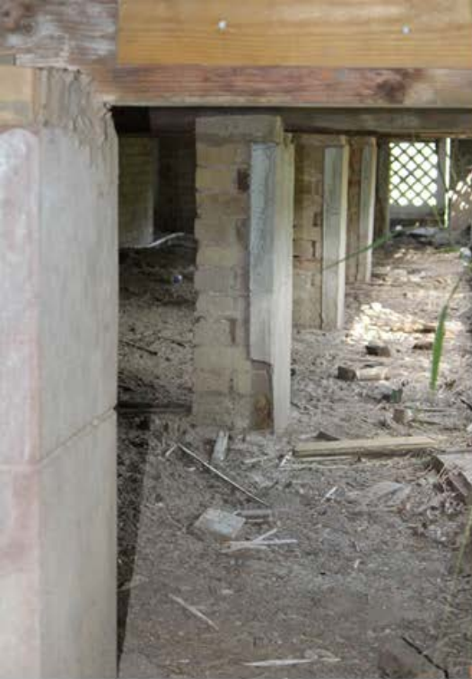
Fig 37. Bypassed original porch piers left after porch was extended three feet.
