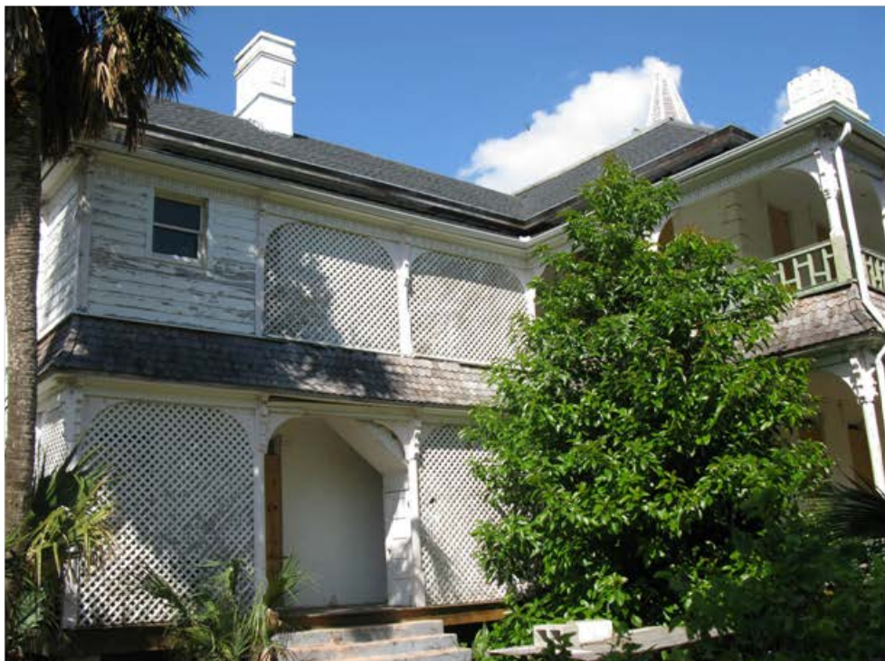
Fig 39. Second floor porch on southwest corner enclosed to accommodate a small bathroom.
