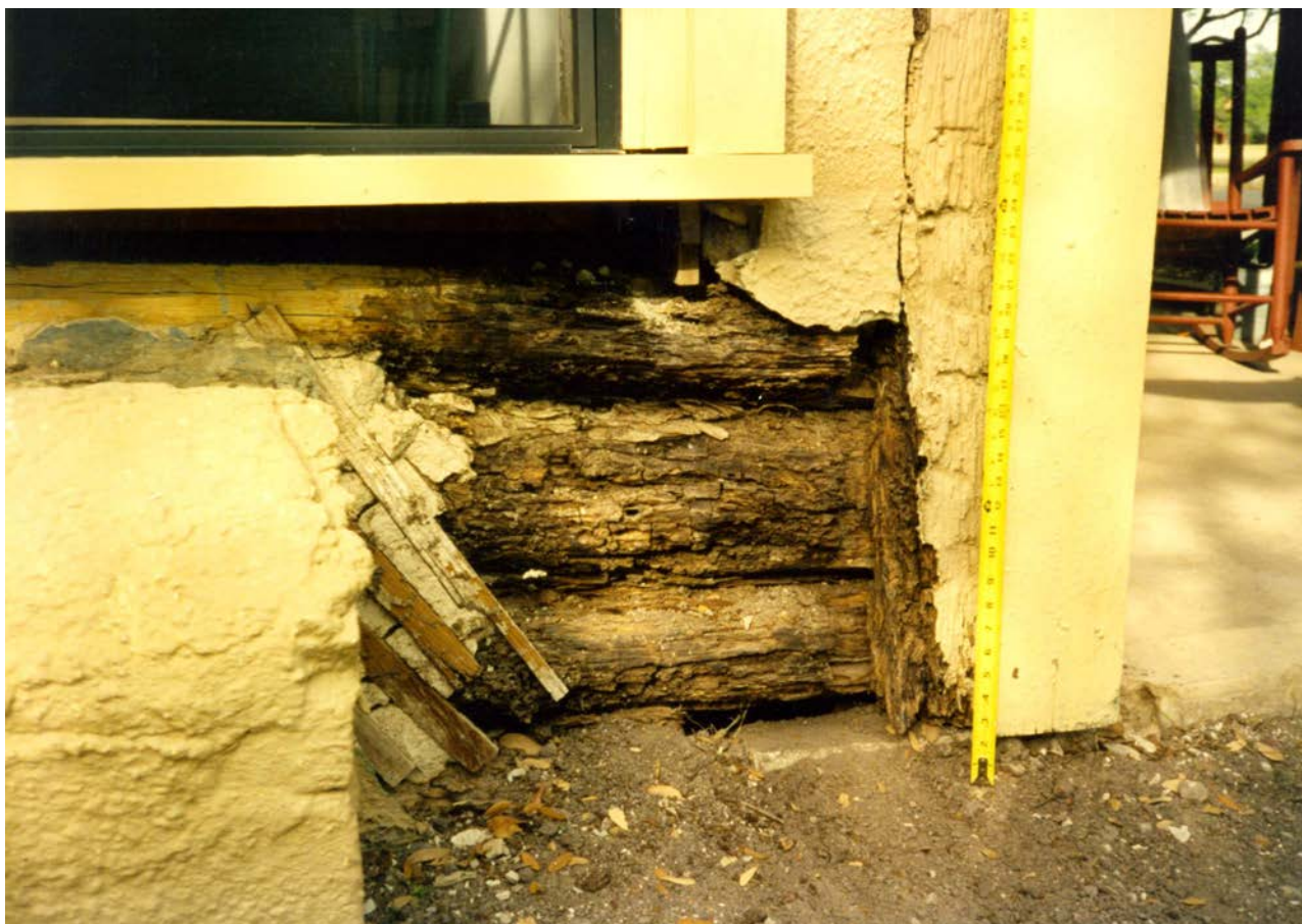
SOUTHEAST CORNER OF QUARTERS No. 4 , 1996. Re-plastering exposed original 1854 construction of vertical posts and horizontal logs. Water damage was mitigated by re-plastering.
