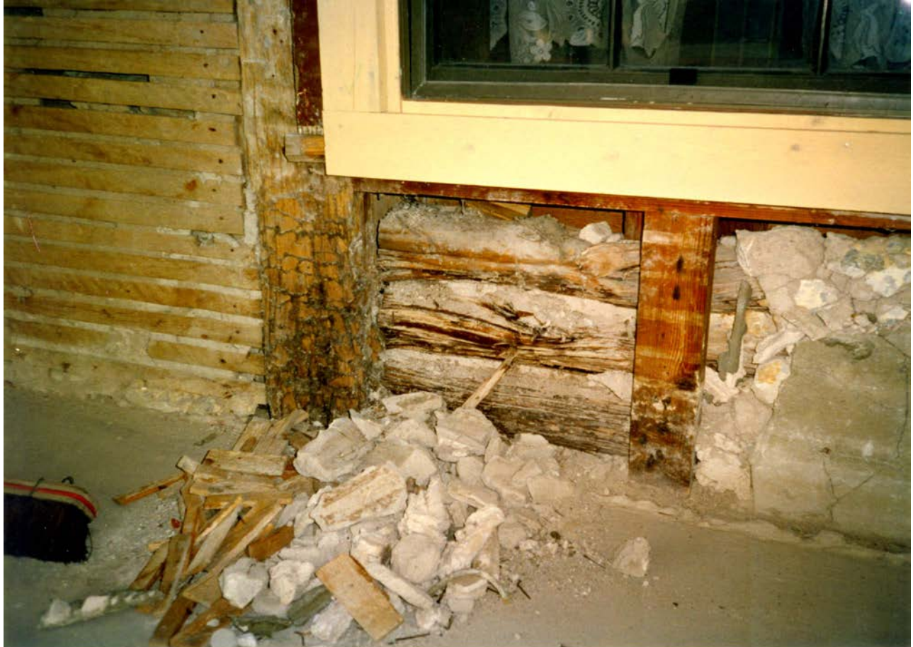
FRONT PORCH OF QUARTERS No. 4, 1996. Re-plastering exposed original 1854 construction of vertical posts and horizontal logs.
