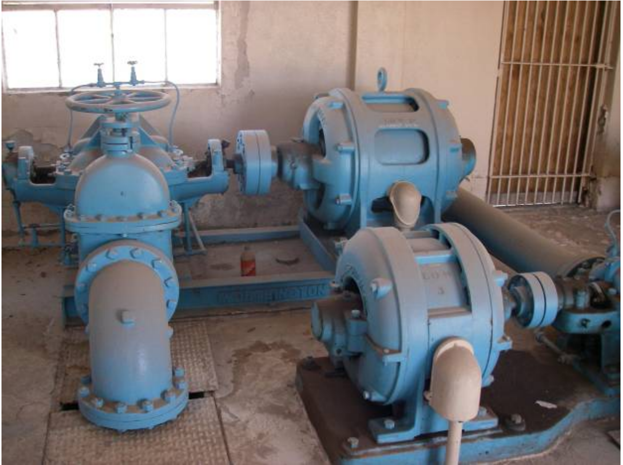
Figure 7. Equipment inside the main building. Photograph by Stephanie Katauskas.
