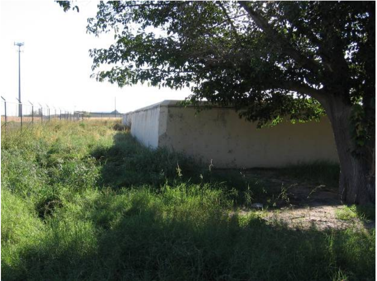
Figure 9. Rear (north) of settling basins, camera facing east. Photograph by Summer Chandler.
