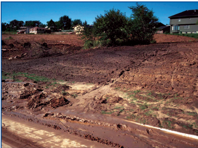
Figure 1. Nonpoint source pollution: sediment runoff pollution from a construction site (Photo courtesy of USDA NRCS)
