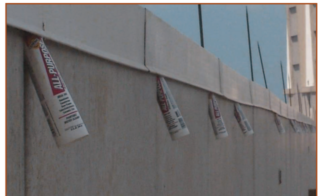
Figure 12. In long areas, place eviction tubes about 6 feet apart along the entire distance to enable all the bats to exit. (Source: Fly By Night Inc.)
